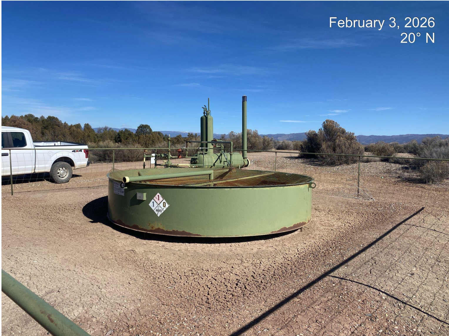
Photo 3. View of produced water secondary containment berm which is insufficient.
