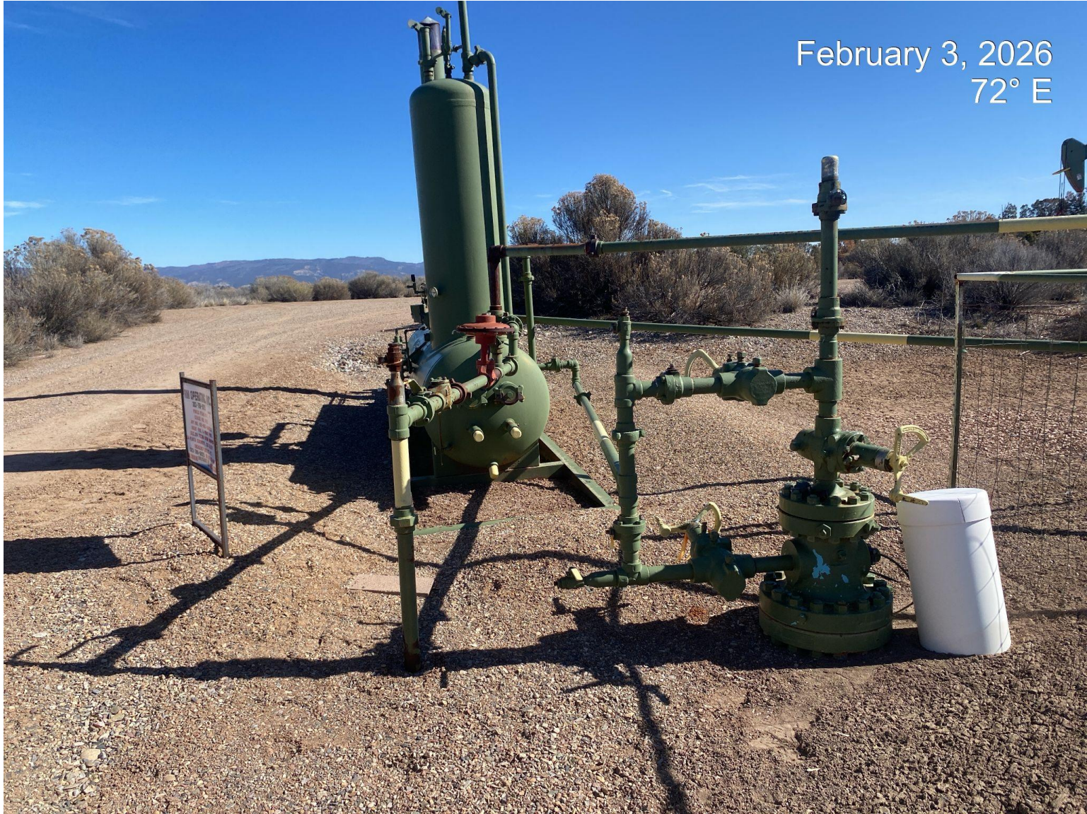
Photo 2. View of wellhead assembly.
