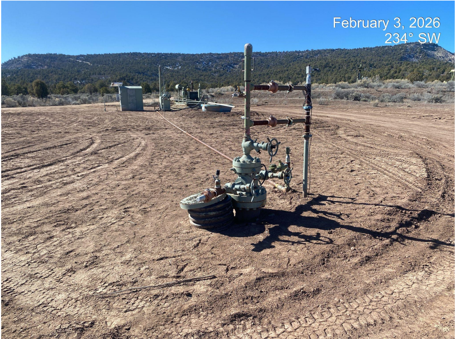
Photo 2. View of wellhead.
