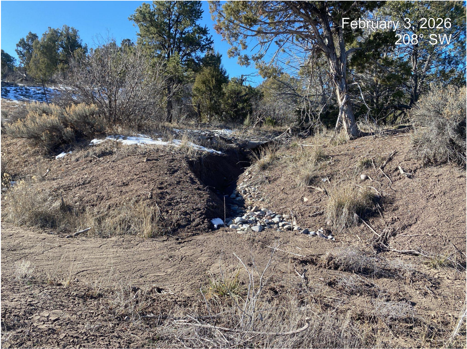
Photo 2. Gully erosion persists in the southern cut slope.
