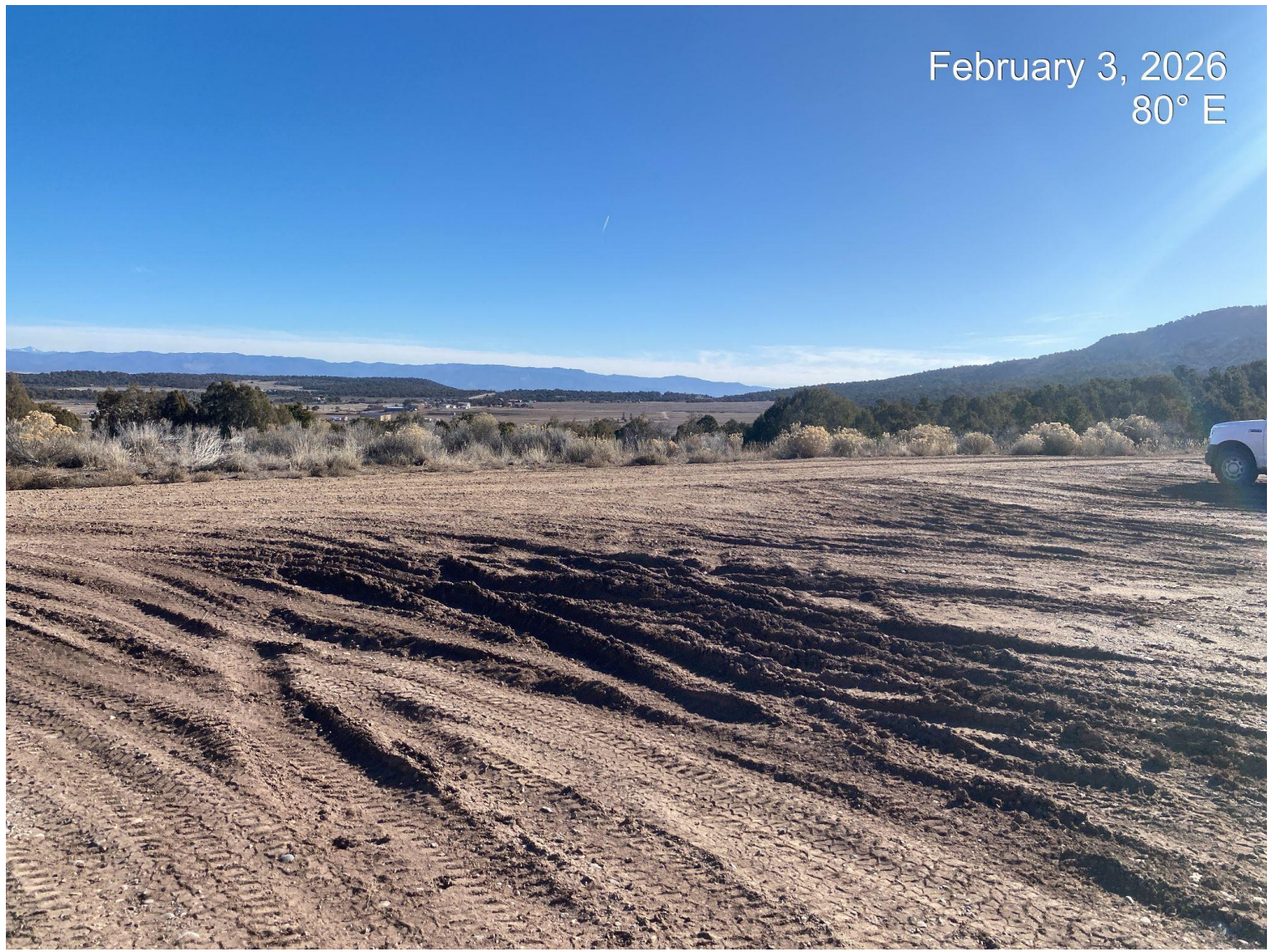
Photo 5. Rutting forming on the active pad.
