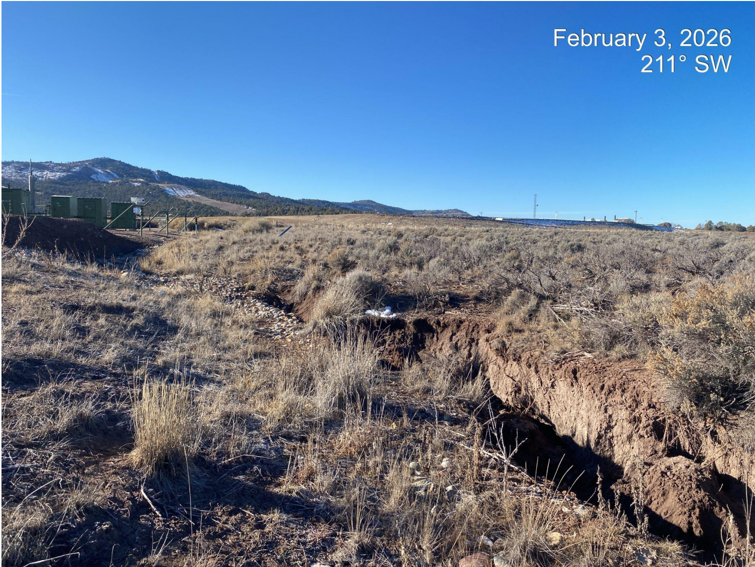
Photo 3. View of gully erosion that has formed in the NW corner of the pad. Gully erosion has formed a long channel running north to a stock pond. Current stormwater BMPs are lacking or insufficient.
