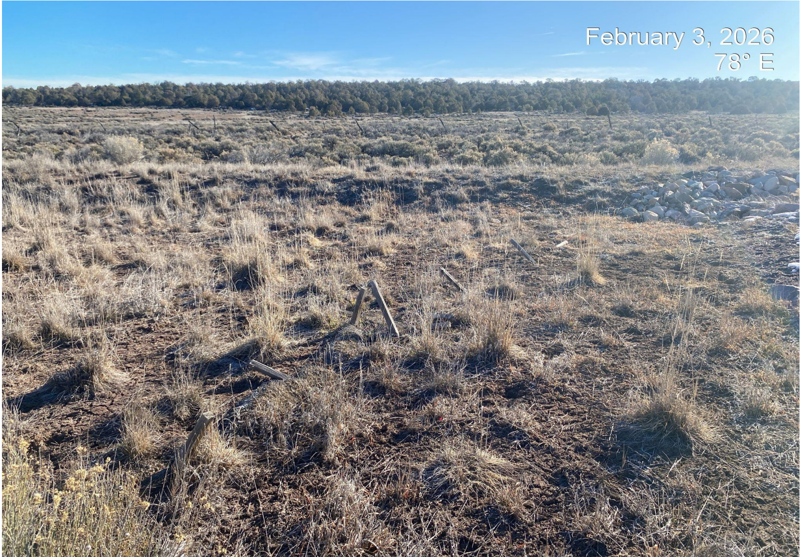
Photo 4. View of wattles and old stakes on the northern edge of the pad.
