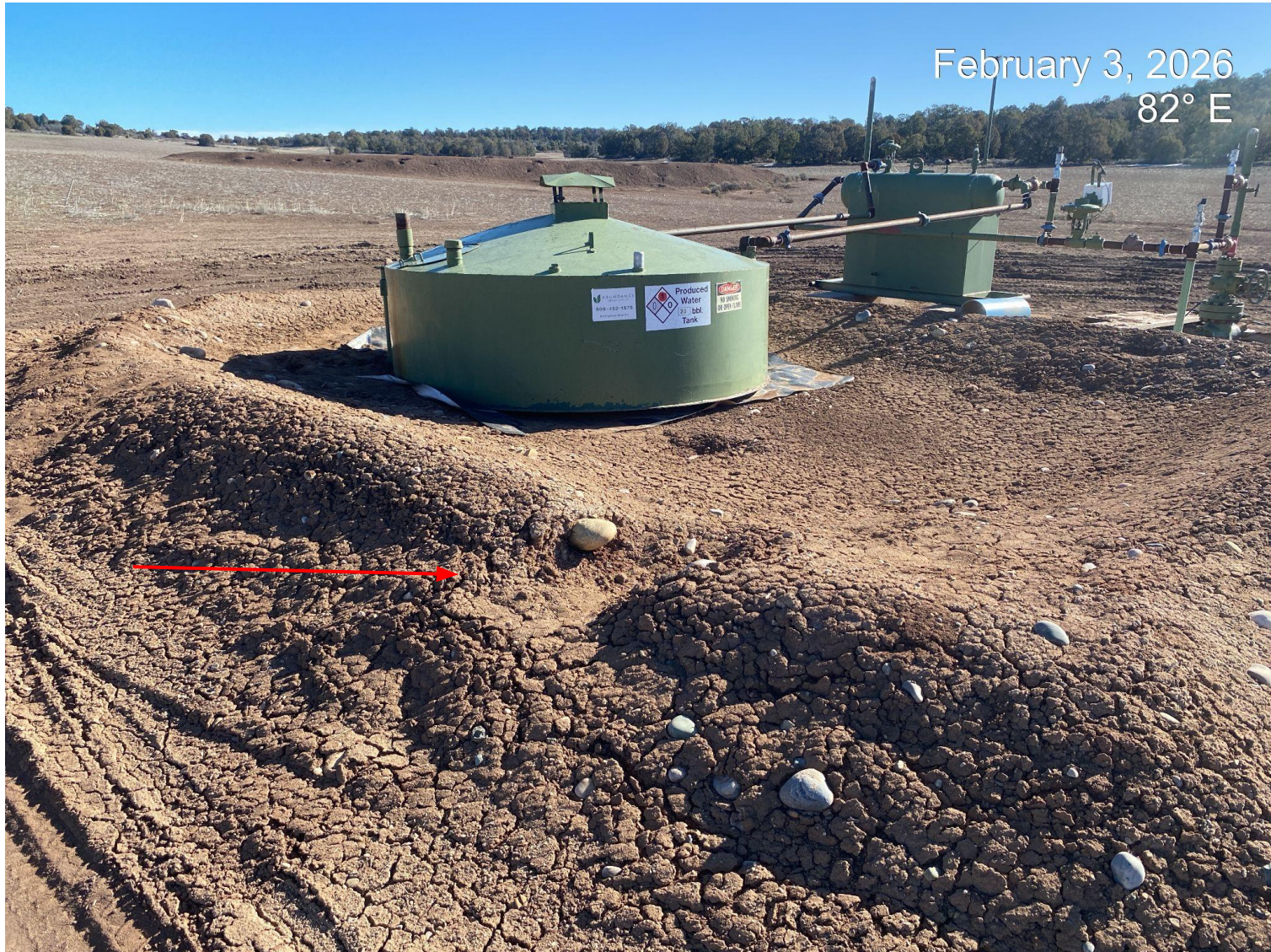
Photo 4. Produced water tank secondary containment berm damage (highlighted with red arrow).
