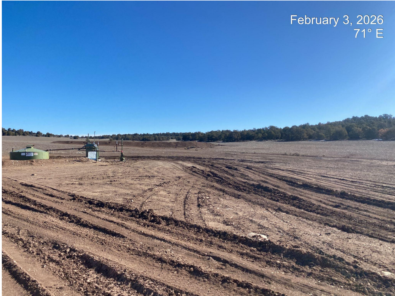
Photo 1. View of the active pad taken from the western edge facing center.
