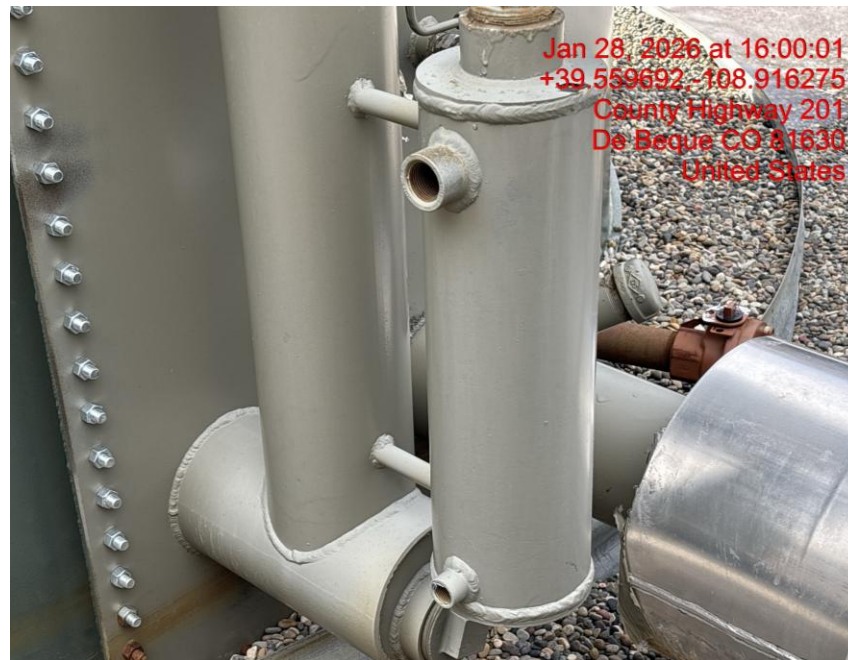
Open-Ended Lines on Tank Burner – Photo #02555
