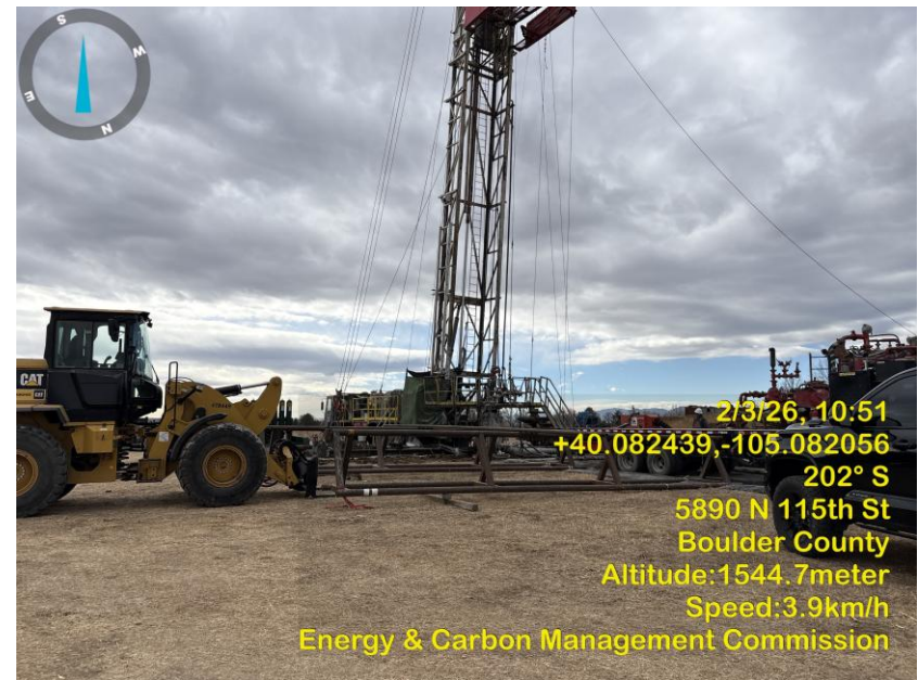
Photo 4 Rig floor, front end loader, pipe racks.
