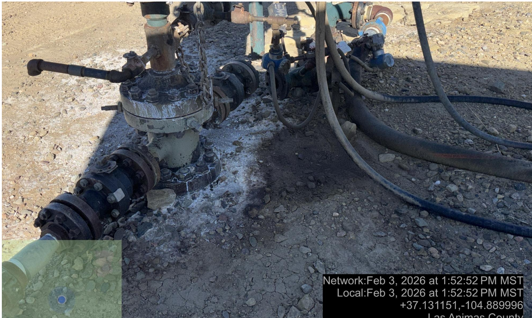
PHOTO 5: AREA OF IMPACTED SOIL AROUND WELLHEAD BOTH OILY STAINING AND WHITE CHALKY MINERAL BUILDUP FROM REPEATED WELL PACKING LEAKING. Conduct maintenance on equipment, cleanup stained material and review self inspection processes. COMPLY WITH RULE 1002,.(2).D. CA DATE 2-10-2026.
