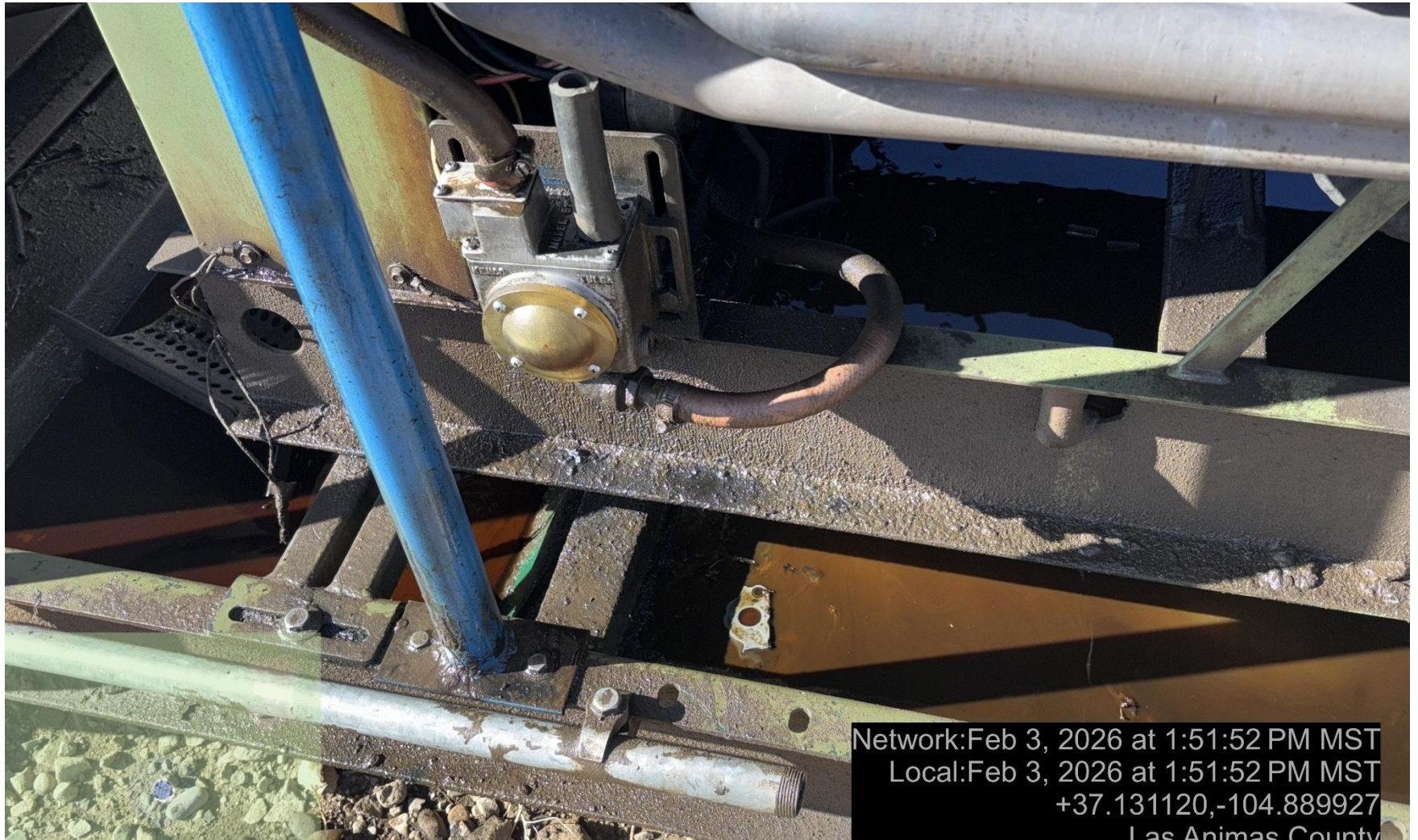
PHOTO 6: OILY WASTE IN PRIME MOVER SKID DOES NOT APPEAR TO BE FROM LEAKING EQUIPMENT, IT APPEARS THAT THE OIL FROM THE ENGINE HAS BEEN DRAINED INTO SKID WITH NO WILDLIFE PROTECTION SCREEN OR NETTING. STOP DRAINING ENGINE OIL INTO SKIDS WITH NO WILDLIFE PROTECTION, DRAIN OIL PER RULE 1002..(2).D & 1002.f.(2)B, Comply with general provisions of the oil and gas act for wildlife protection AND SB-181. CA DATE 2-4-2026.
