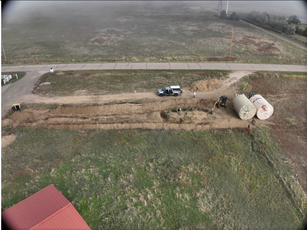
In View – Tank Battery, Separator, Flowlines
