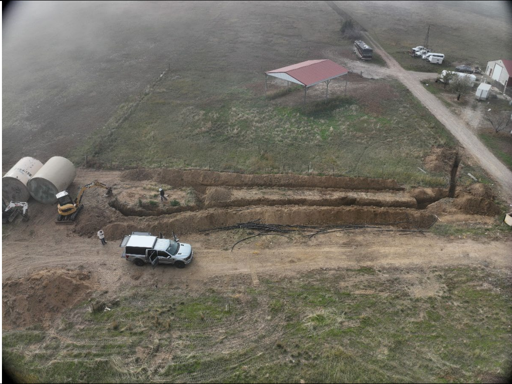
In View – Tank Battery, Separator, Flowlines
