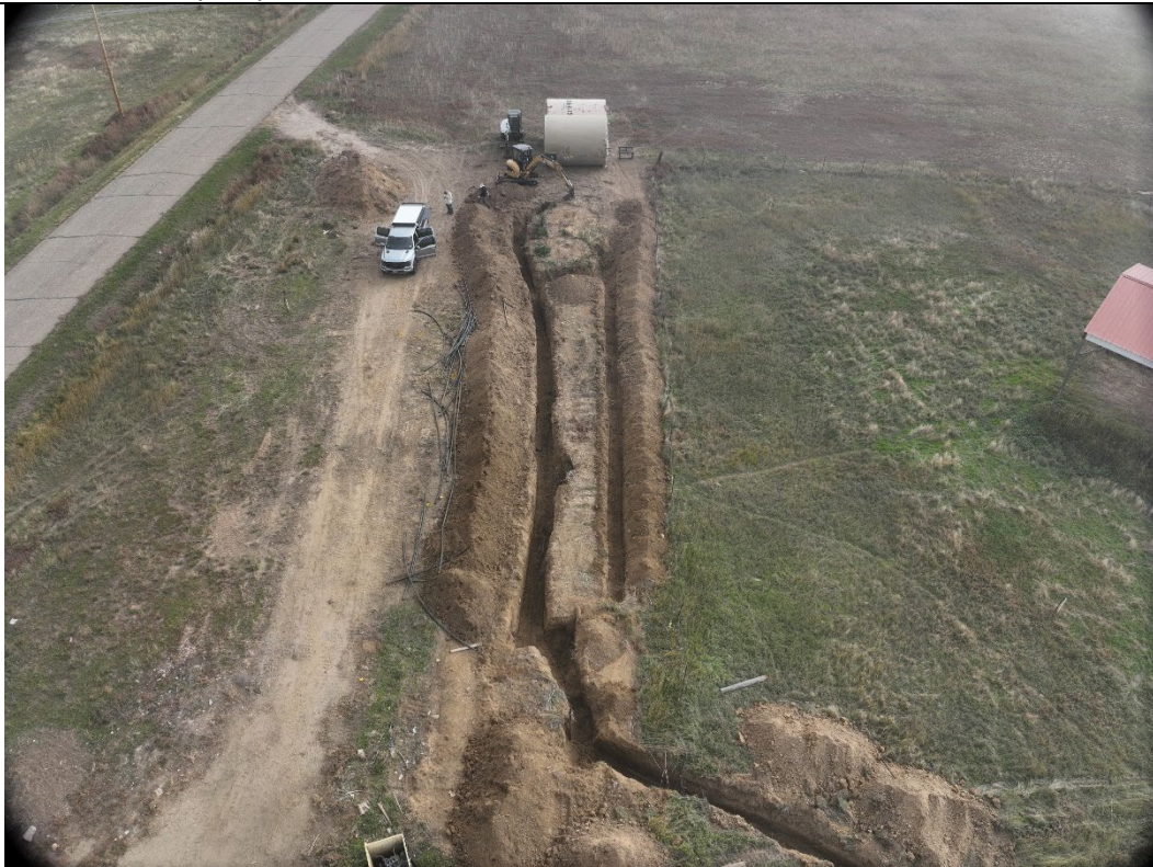
In View – Tank Battery, Separator, Flowlines
