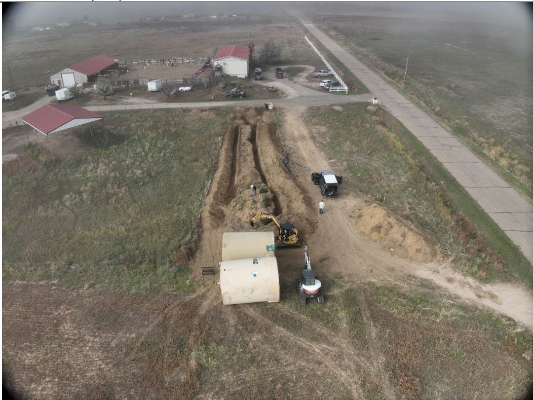
In View – Tank Battery, Separator, Flowlines
