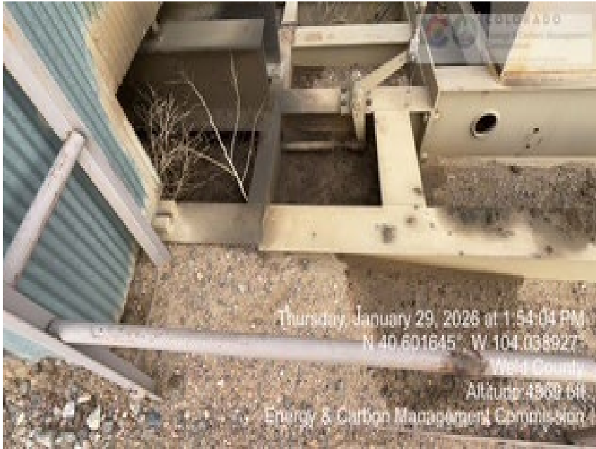
Photo 3 – Pumping Unit – Stained Soil
