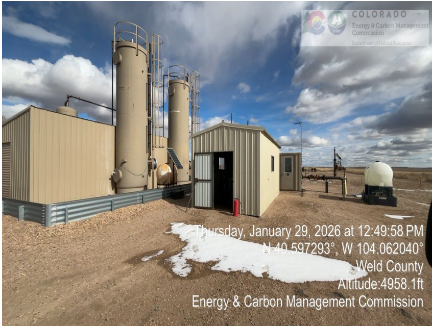
Photo 23 – Heater Treaters and Compressor
