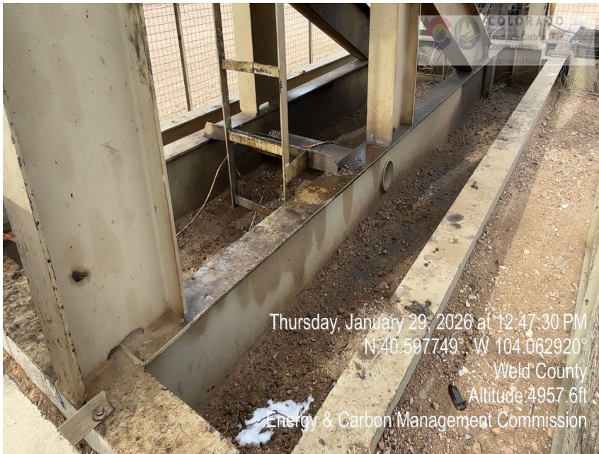
Photo 13 – 2-6H Pumping Unit – Stained Soil
