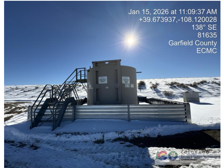
Photo # 1078 Tank battery lacks signage/not in compliance with CECMC rules
