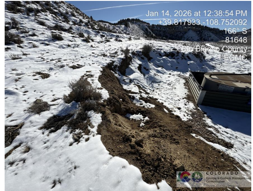
Photo # 1054 Erosion & transport of sediment on cut slope, sediment is migrating onto location near tank battery, the cut slope has experienced progressive erosion and is now actively sloughing, resulting in slope instability.
