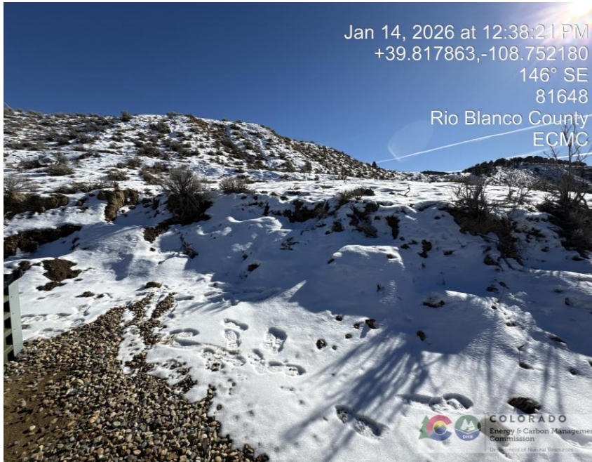
Photo # 1052 Erosion & transport of sediment on cut slope, sediment is migrating onto location near tank battery, the cut slope has experienced progressive erosion and is now actively sloughing, resulting in slope instability.
