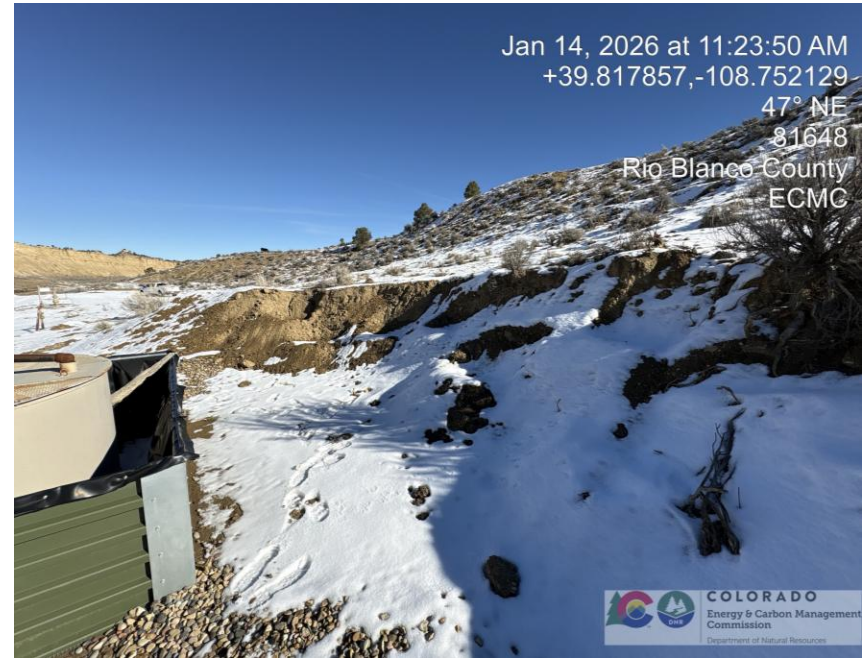
Photo # 1006 Erosion & transport of sediment on cut slope, sediment is migrating onto location near tank battery, the cut slope has experienced progressive erosion and is now actively sloughing, resulting in slope instability.
