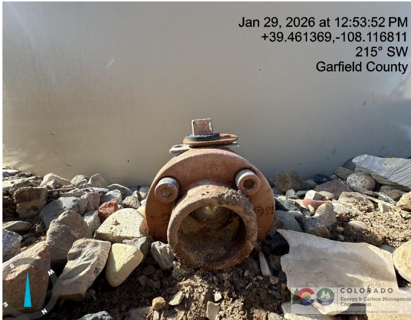
Photo # 7275 Open ended load line
