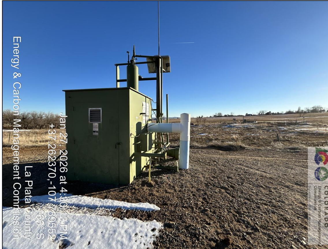
13. Meter run and vertical heated separator. Bird protector on heater exhaust stack.
