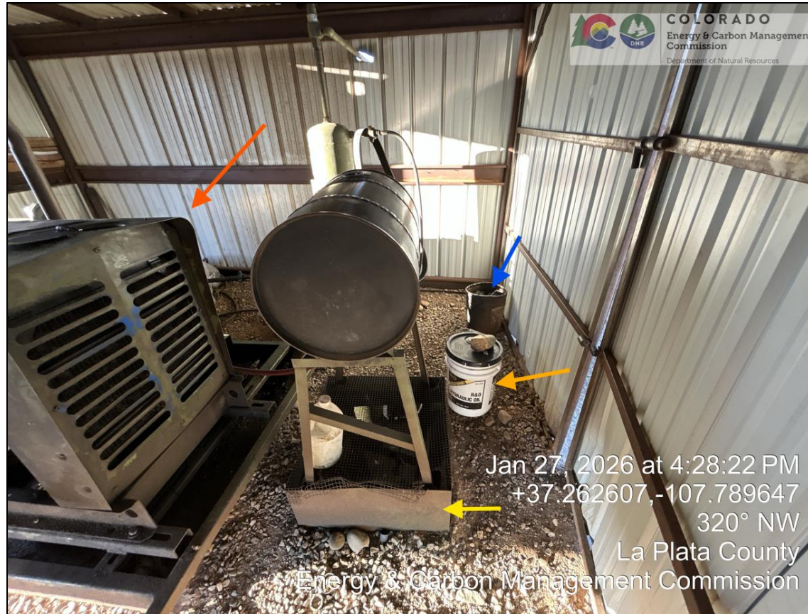
09. View inside hydrostatic drive pump shed. There is lube or secondary hydraulic oil reservoir atop a secondary containment structure that is \frac{3}{4} full (yellow arrow indicates level), a bucket of hydraulic oil (orange arrow), an open-topped bucket with oily rags (blue arrow), and various unused hoses, pipe fittings and other equipment behind the motor (red arrow). There gravel on the ground has oil stains. There is also an unlabelled jug and oil stains on the gravel in various place.
