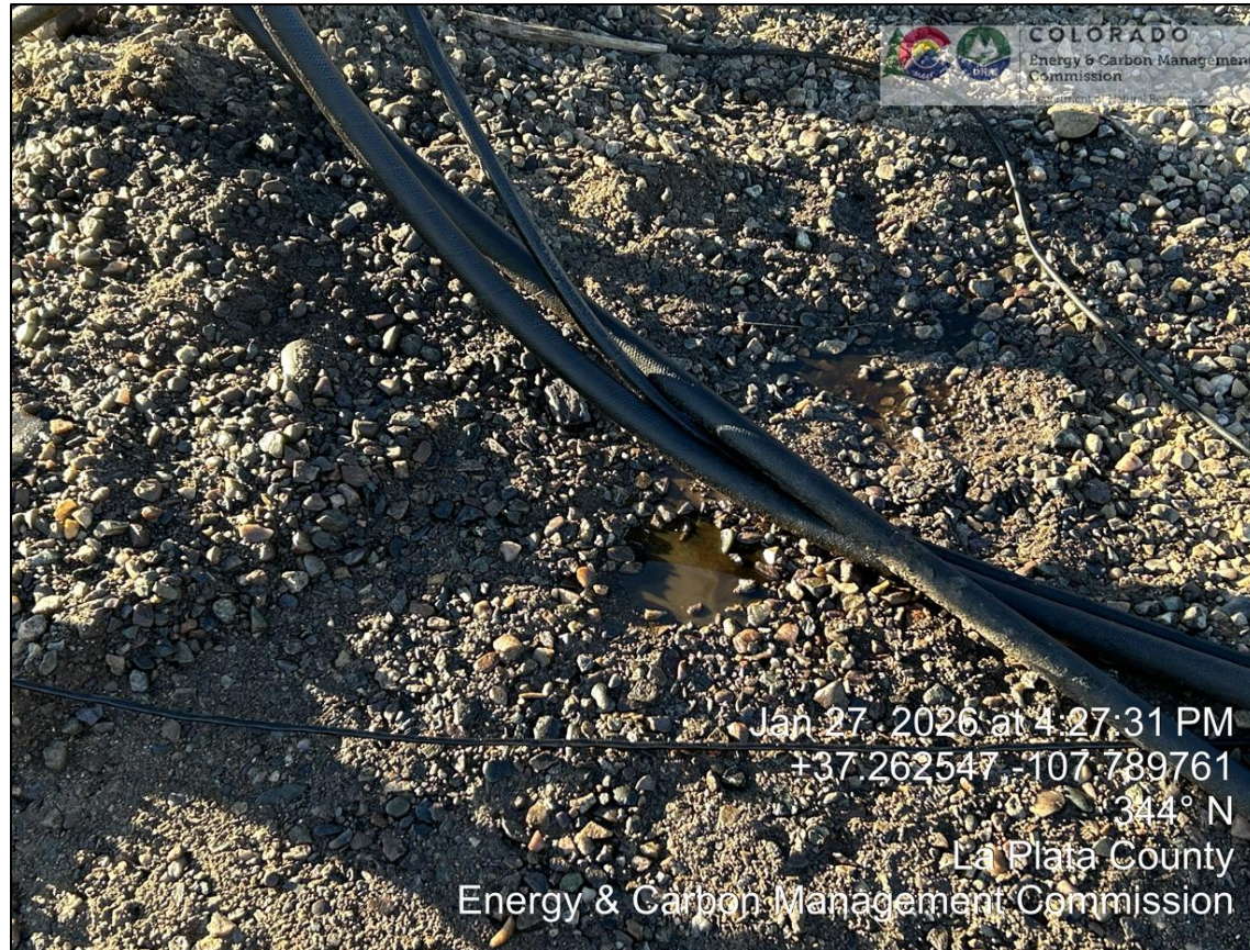
06. Puddle of free-standing hydraulic fluid by wellhead indicating ground saturation. Hoses are for the hydraulic drive unit.
