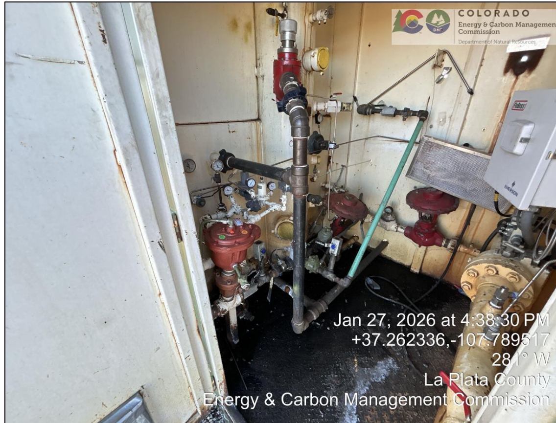
12. View inside meter run shelter. Mineral precipitate on ground is consistent with produced water leakage. Last meter calibration date: 09/25/2025.
