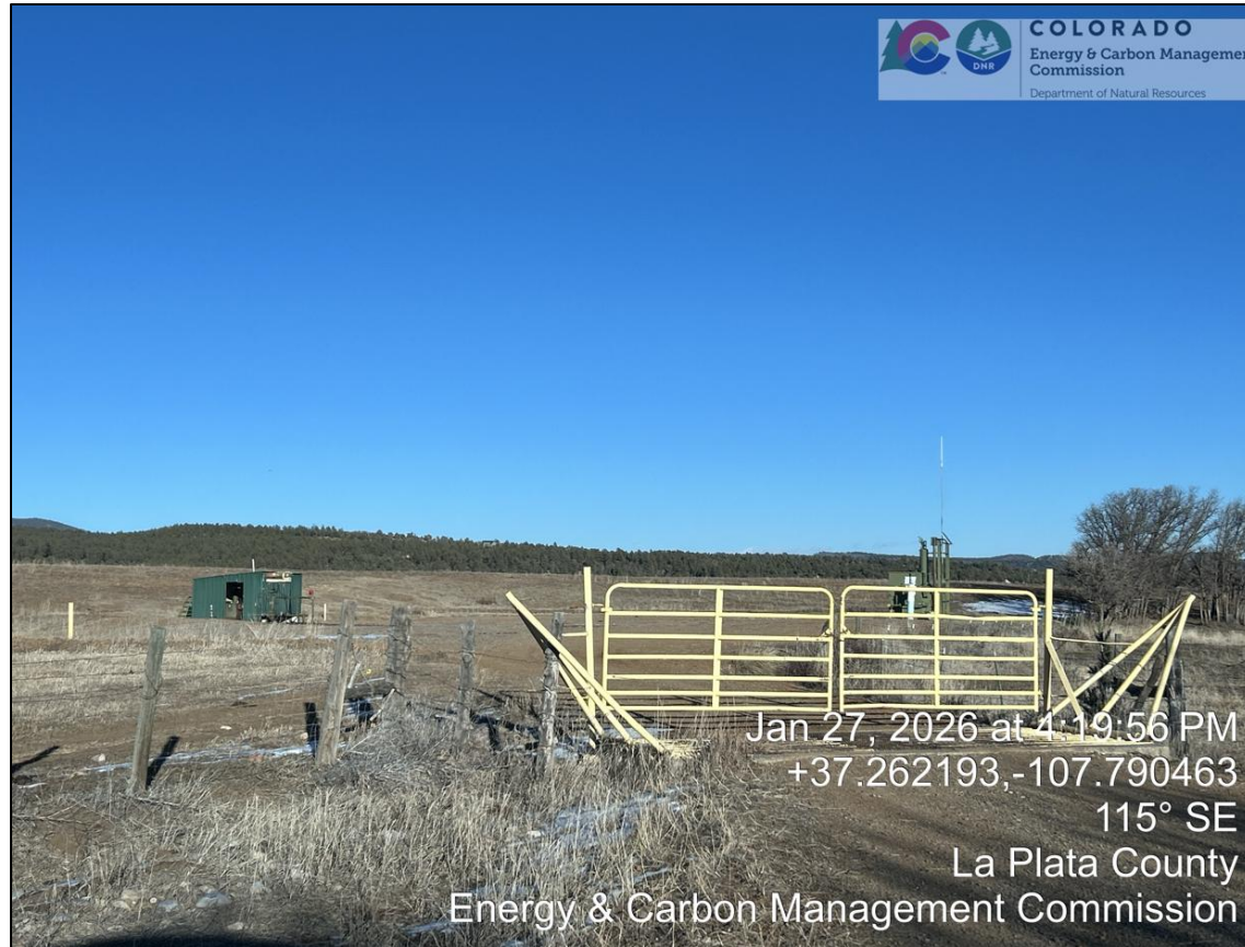
03: Access gate at edge of well pad. No lock.
