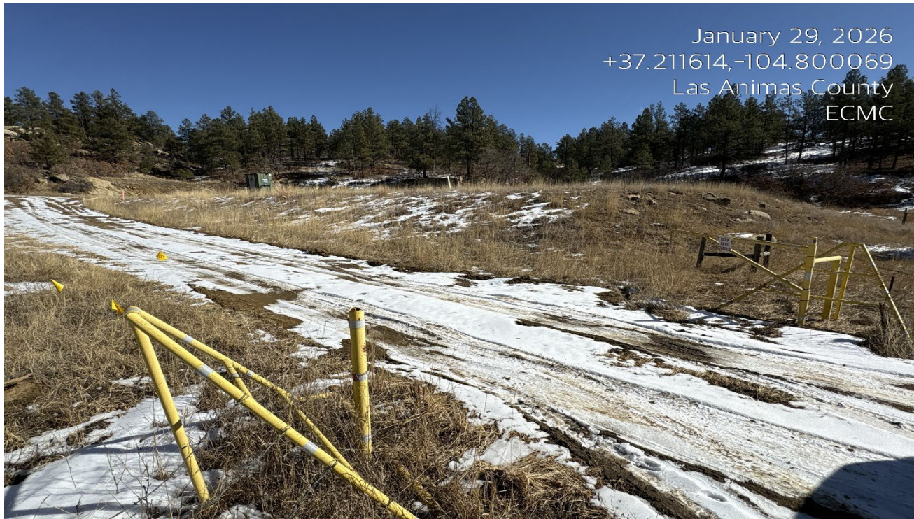
Photo 1. Facing northeast at the access road. The cattleguard is filled in with sediment and needs to be cleaned out.
