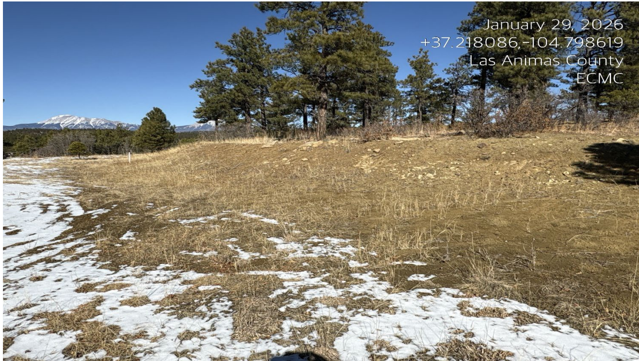
Photo 9. Facing north toward the cut slope. There are some bare areas that could benefit from hand seeding to establish more vegetation.
