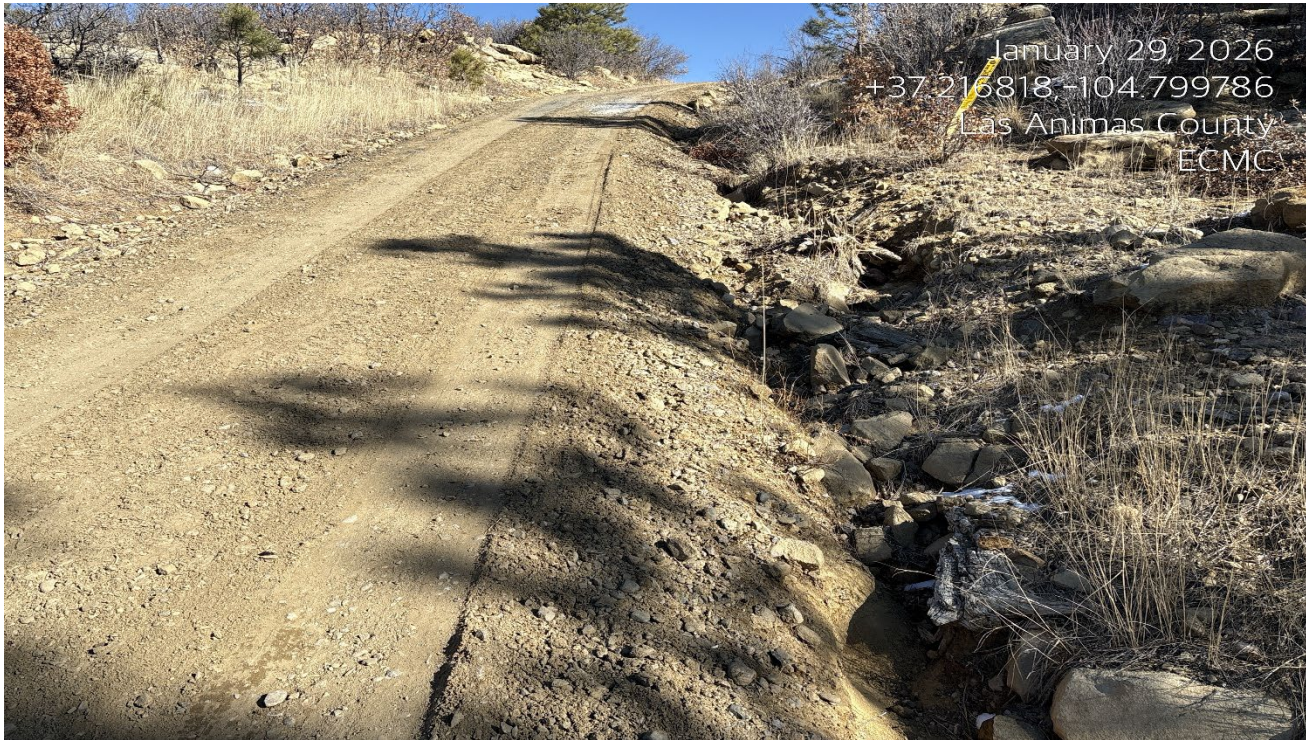
Photo 5. Facing northeast along the access road. BMP's along the roadside will need to be installed. The road has narrowed due to erosion of the roadbase along the road sides.
