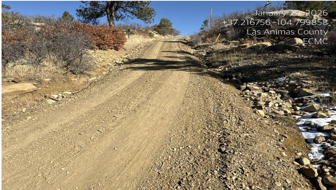
Photo 3. Facing northeast along the access road. There is erosion along both sides of the road that will need to be repaired with BMP's.
