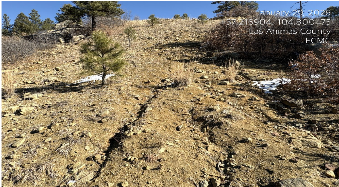
Photo 2. Facing toward the flowline area where erosion has occurred. This area will need to be repaired, reseeded, and stabilized.
