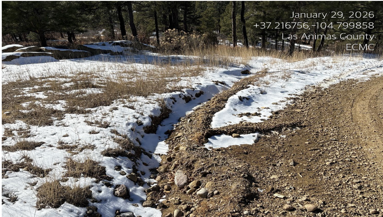
Photo 4. There is a stormwater diversion at the switchback of the road that should have BMP's to prevent erosion such as rip/rap, checkdams. ect.
