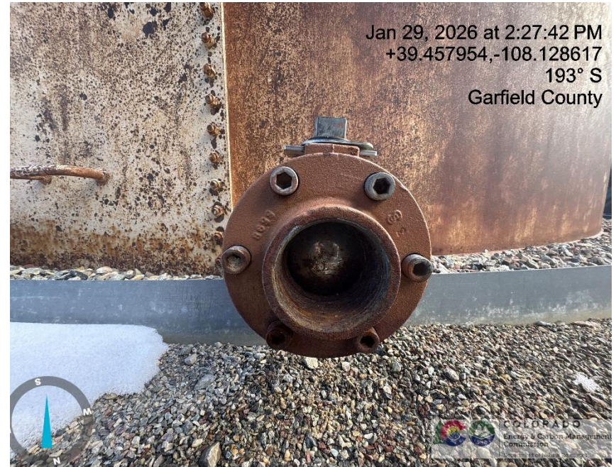
Photo # 7685 Open ended load line
