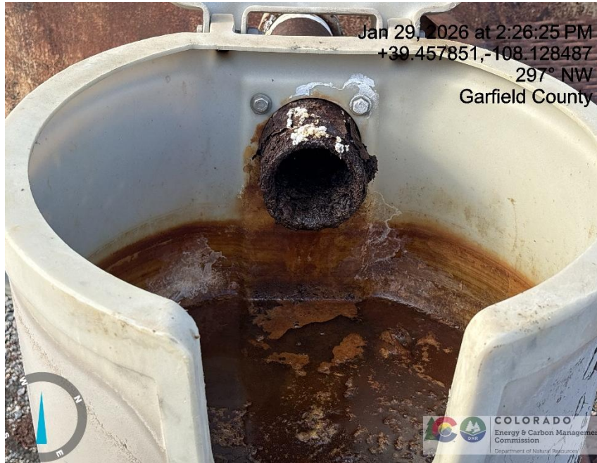
Photo # 7684 Open ended load line
