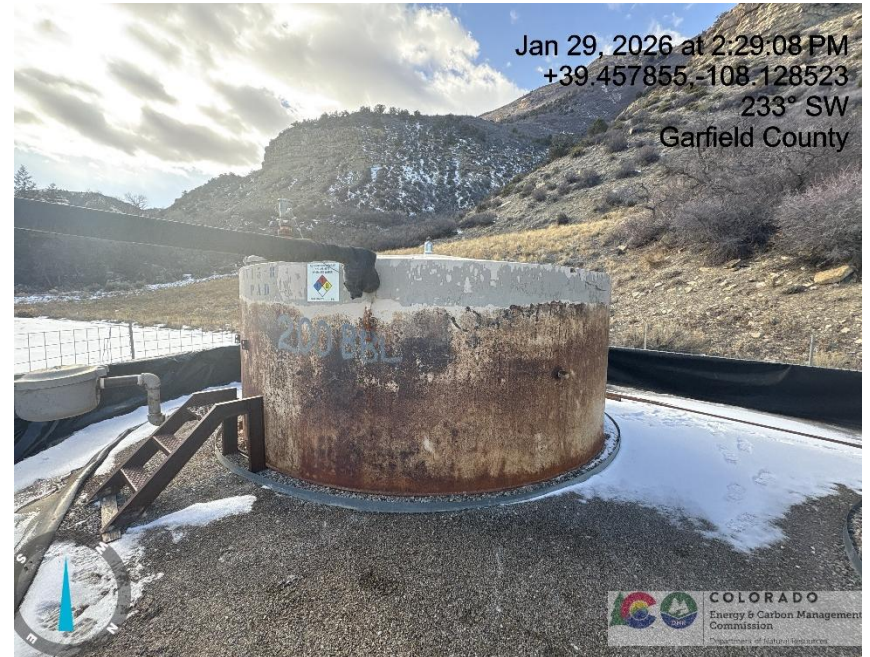
Photo # 7689 Majority of paint has peeled off 200 bbl tank & tank starting to rust
