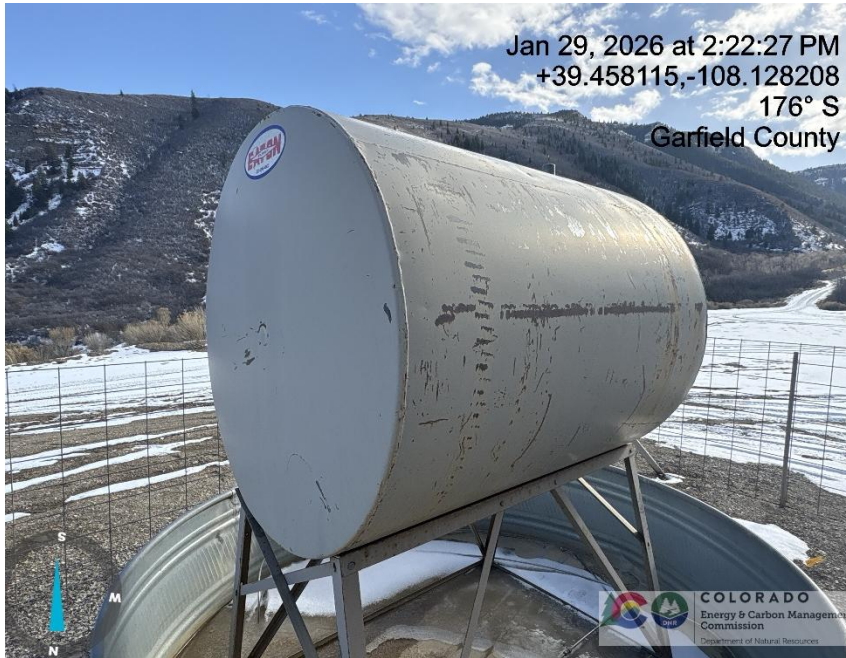
Photo # 7682 Methanol tank
