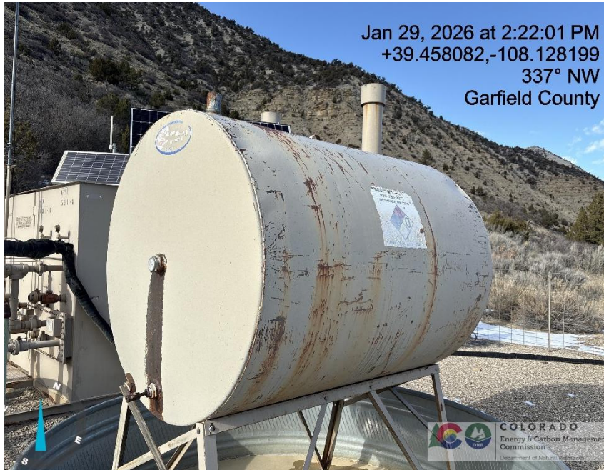
Photo # 7680 Tank label on methanol tank faded & starting to become illegible & label lacks operator name
