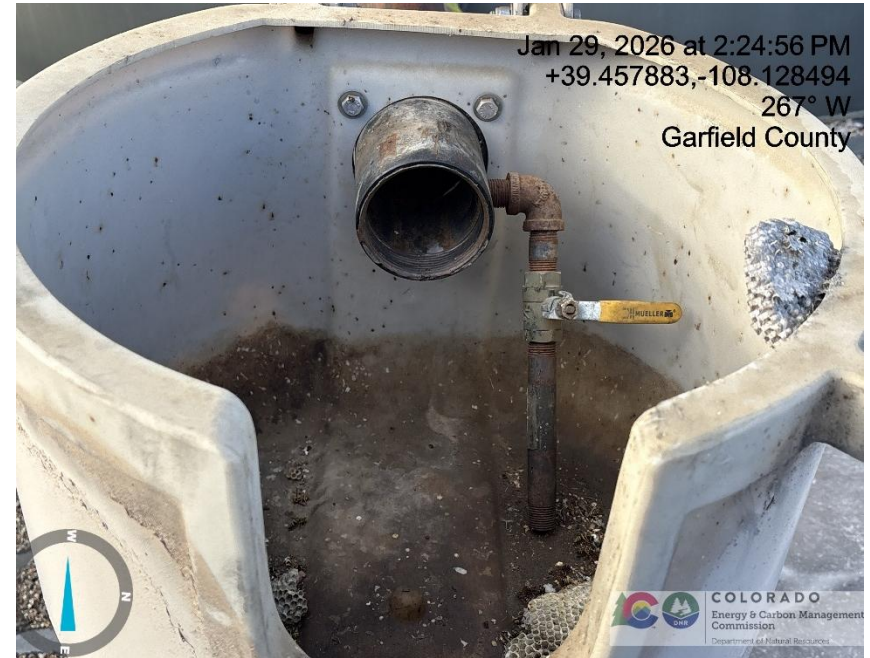
Photo # 7683 Open ended load line
