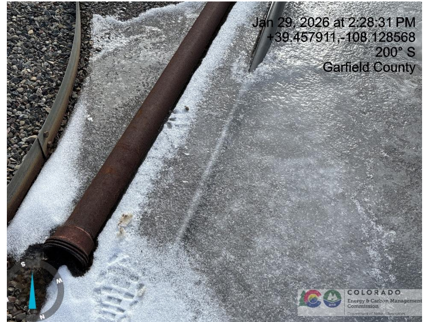
Photo # 7687 Debris in tank battery secondary containment
