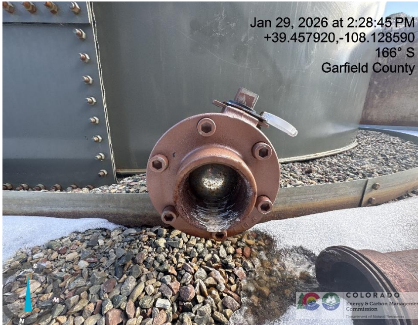
Photo # 7686 Open ended load line
