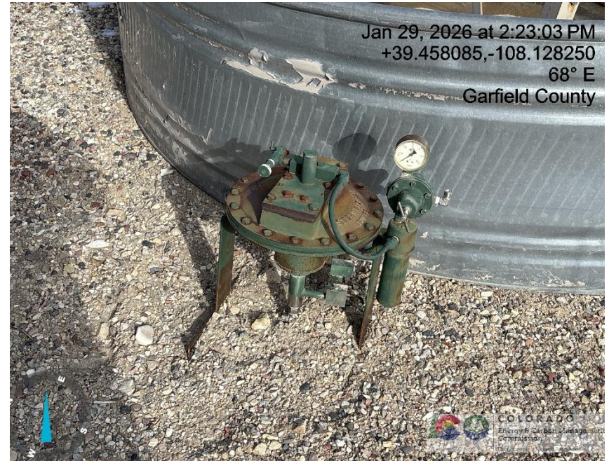
Photo # 7679 Unused western pump near methanol tank
