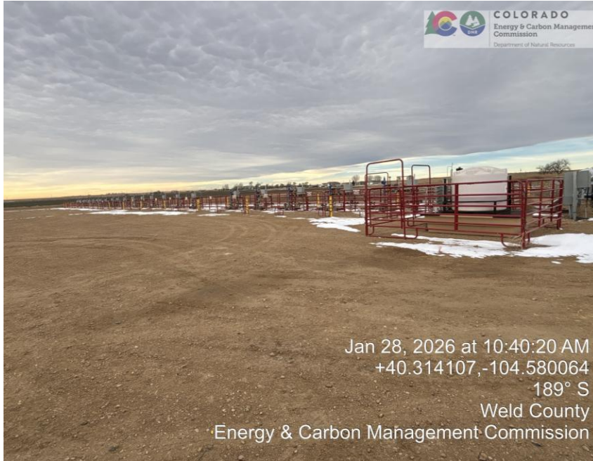
Photo 1 well heads and equipment
