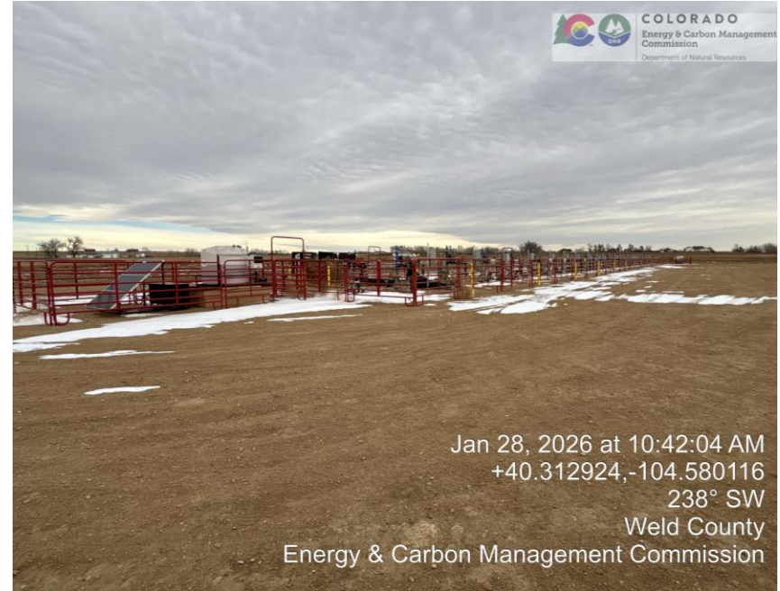
Photo 2 well heads and equipment
