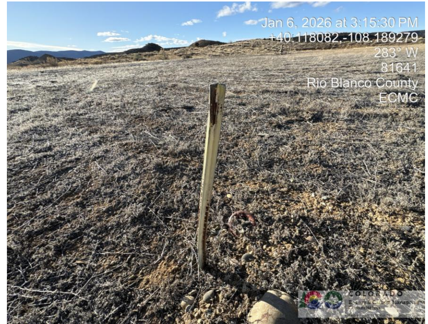
Photo # 0797 1 Improperly marked deadman on west side of location
