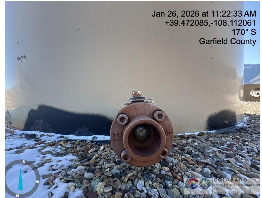
Photo # 4615 Open ended load line
