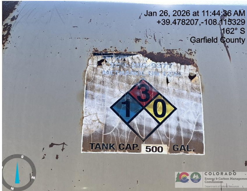
Photo # 4728 Methanol tank label damaged & illegible
