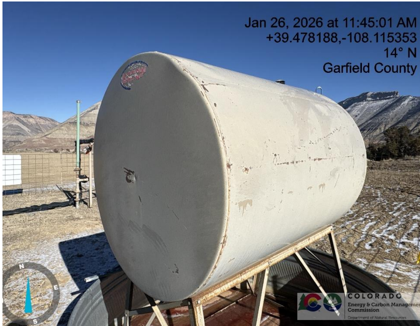
Photo # 4730 Methanol tank
