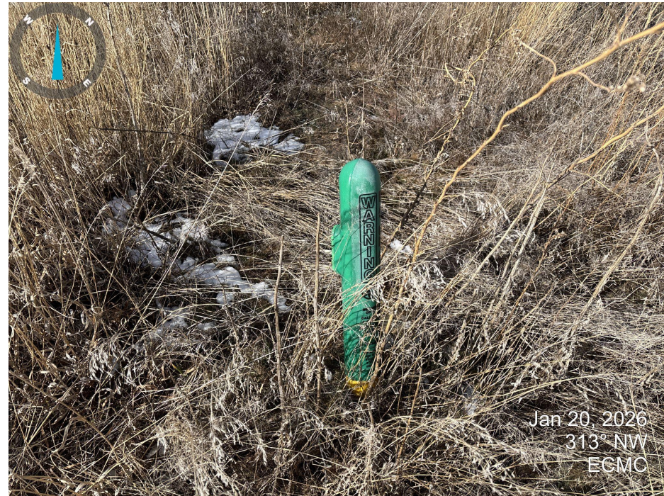
Photo 2. An underground gas line ground test station is present on location. A previous FIRR indicated this may be a permanent piece of equipment. The L shaped vent pipe was not observed on the location.
