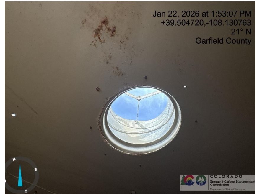
Photo # 4088 Hole in separator/wildlife hazard/available for entry by wildlife
