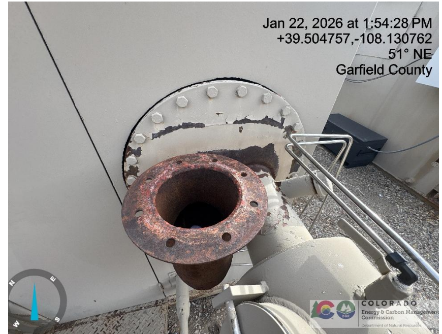
Photo # 4086 Burner exhaust open ended/wildlife hazard/available for entry by wildlife
