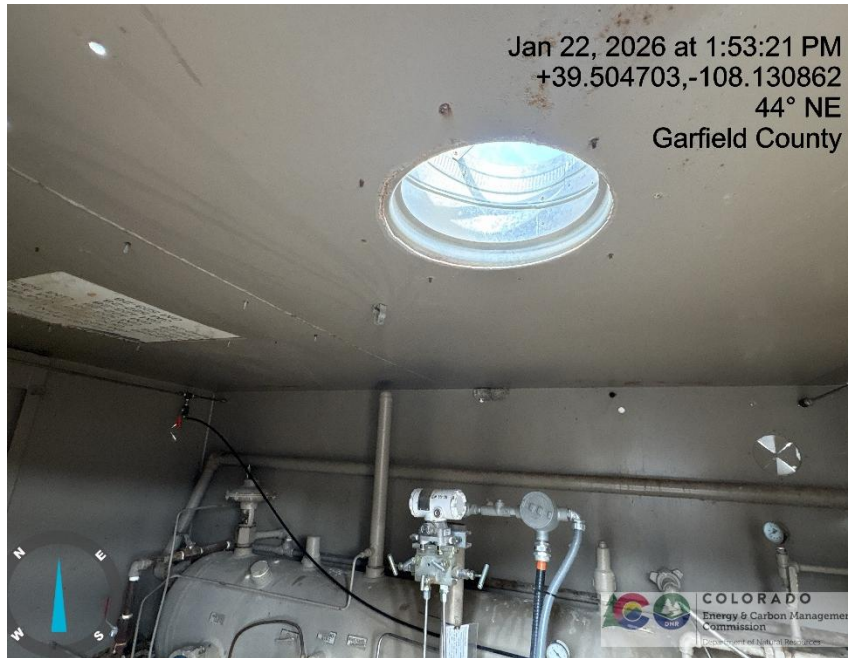
Photo # 4087 Hole in separator/wildlife hazard/available for entry by wildlife
