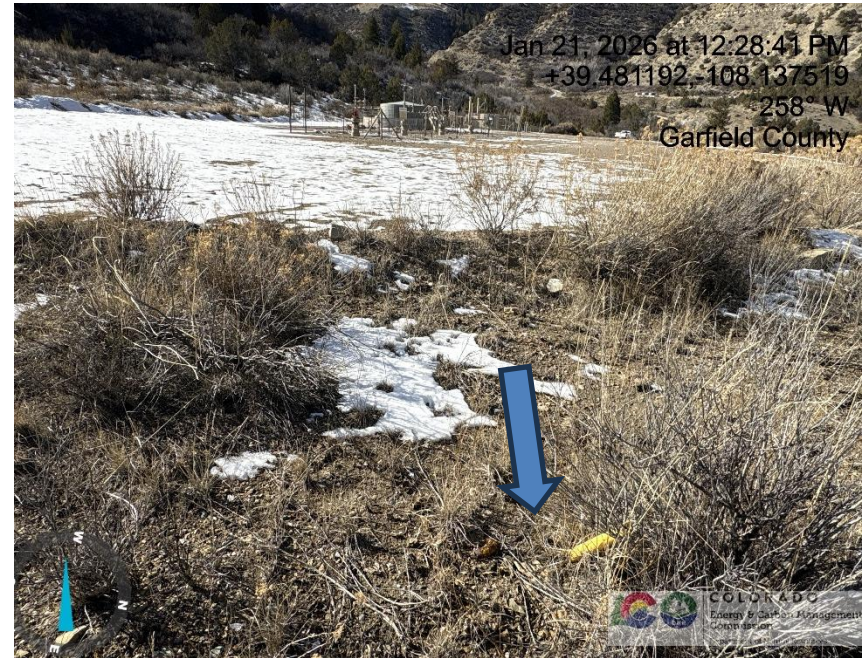
Photo # 3168 Same improperly marked deadman
