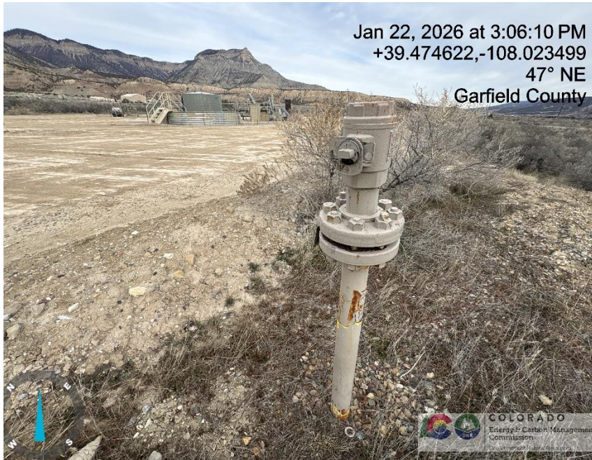
Photo # 4391 Unused flowline lacks lockout tagout (OOSLAT)
