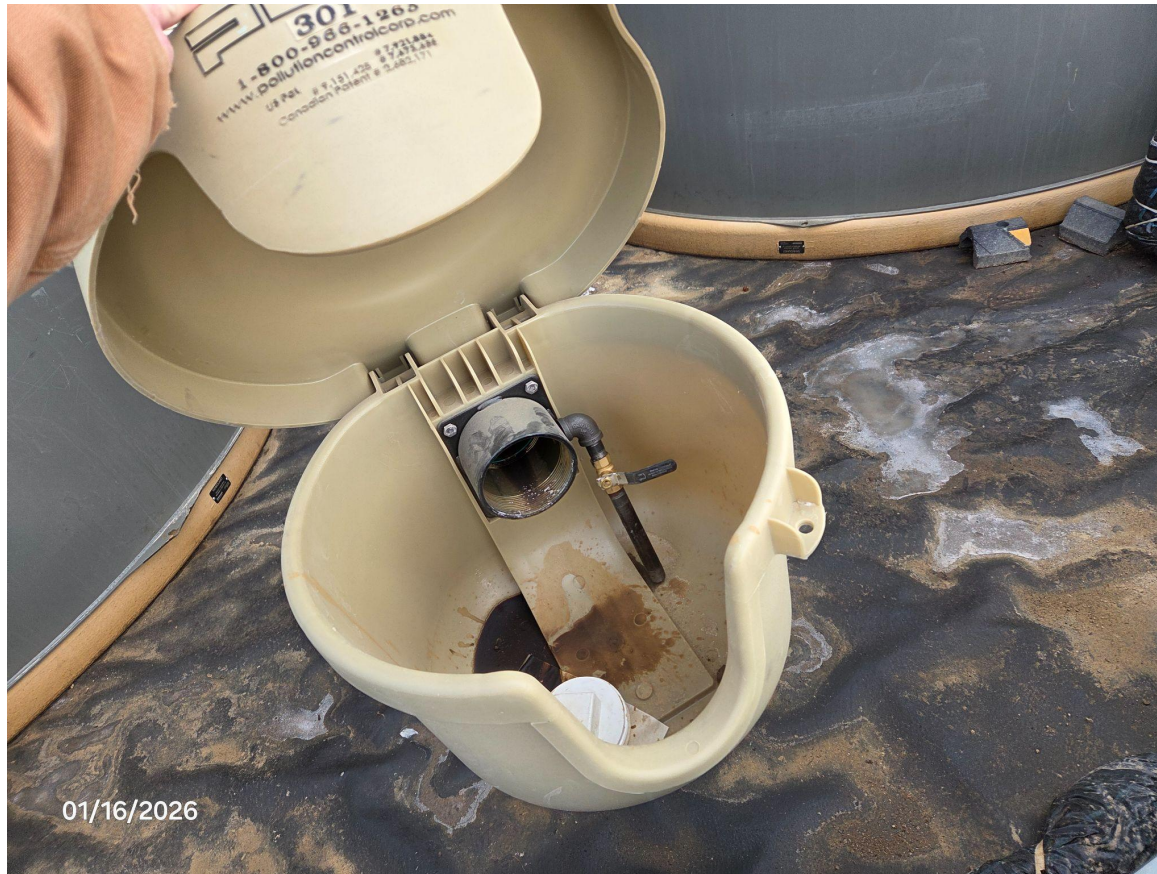
Photo 14: Loadline missing cap/plug.
