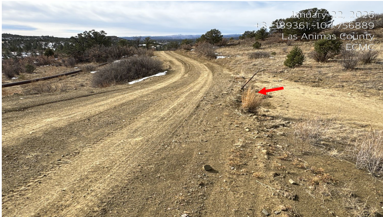
Photo 3. The culvert shown at red arrow has filled in with sediment...
