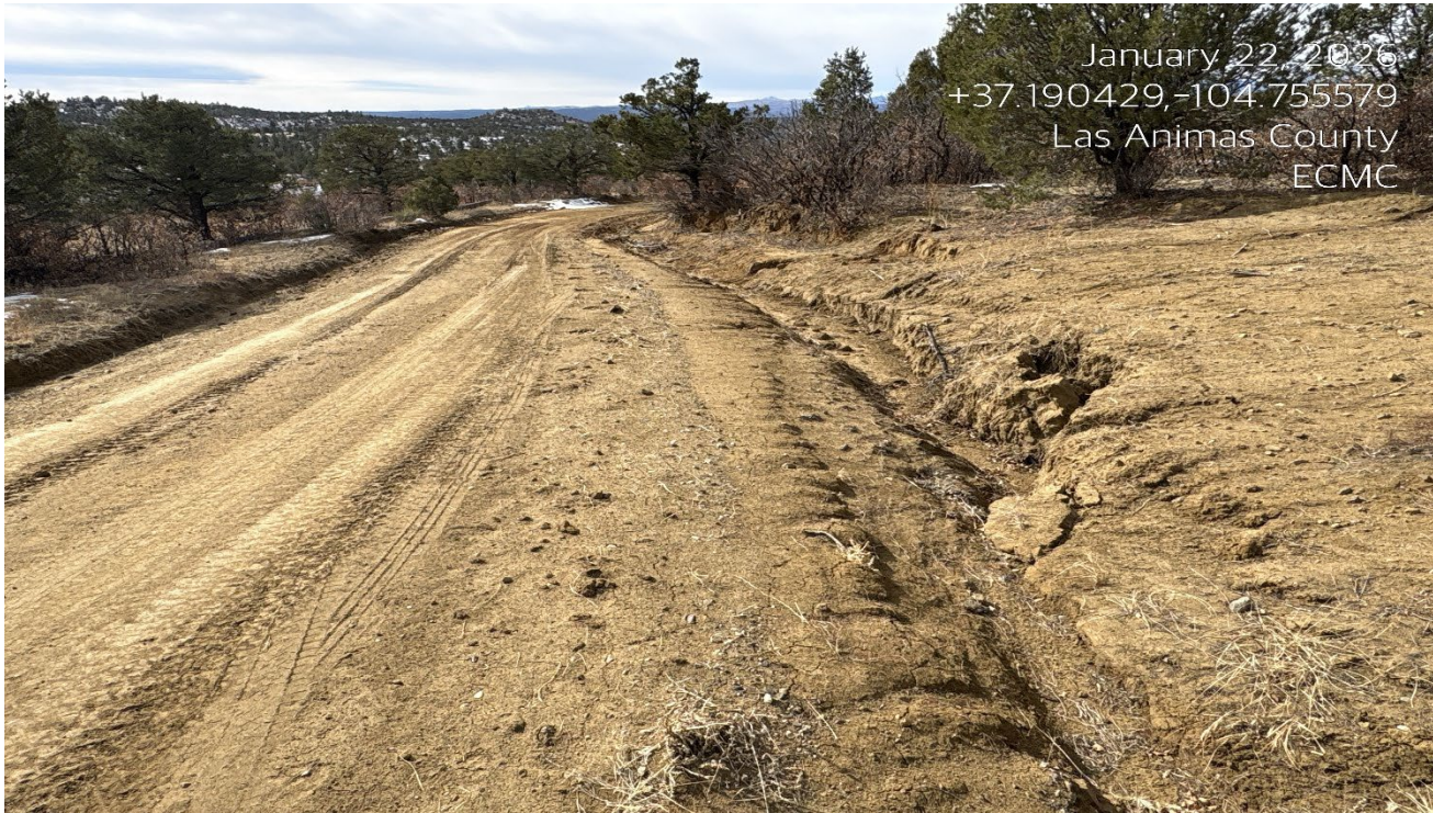
Photo 1. Facing southwest along the main access road which is east of the wellsite. There is erosion along the road and the roadside is not stabilized.
