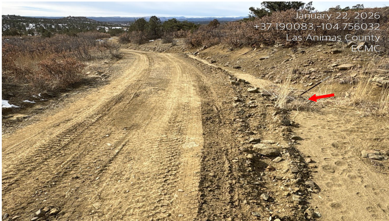
Photo 2. The culvert shown at red arrow has filled in with sediment...
