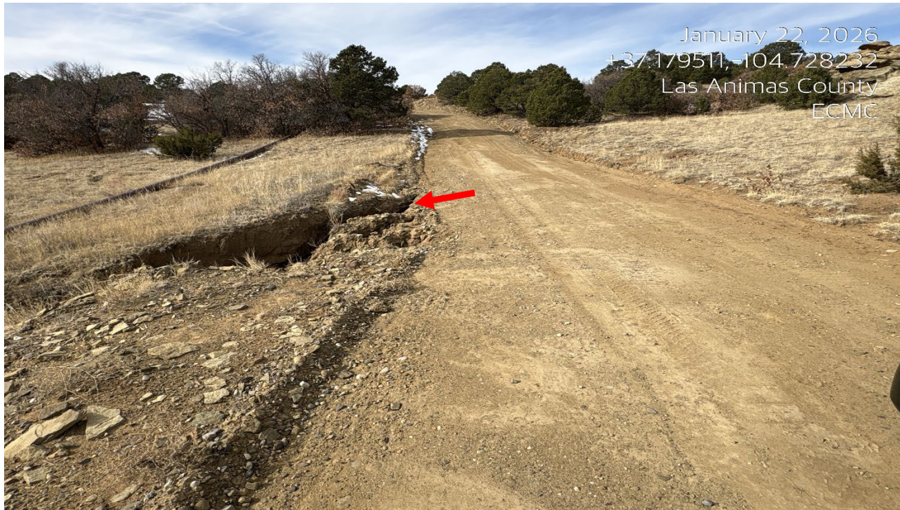
Photo 1. Facing west along the access road. There is an area of erosion shown at red arrow.
