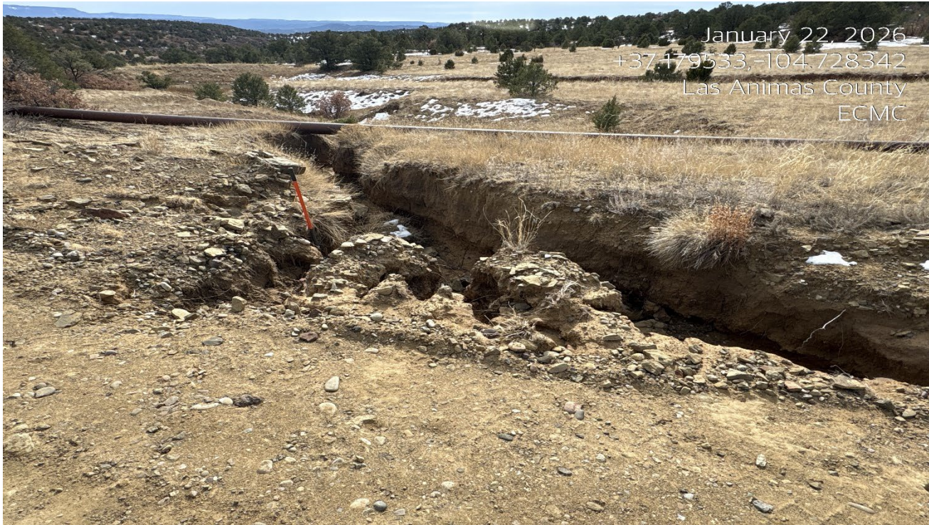
Photo 2. This area of erosion along the roadside will need to be repaired and stabilized..
