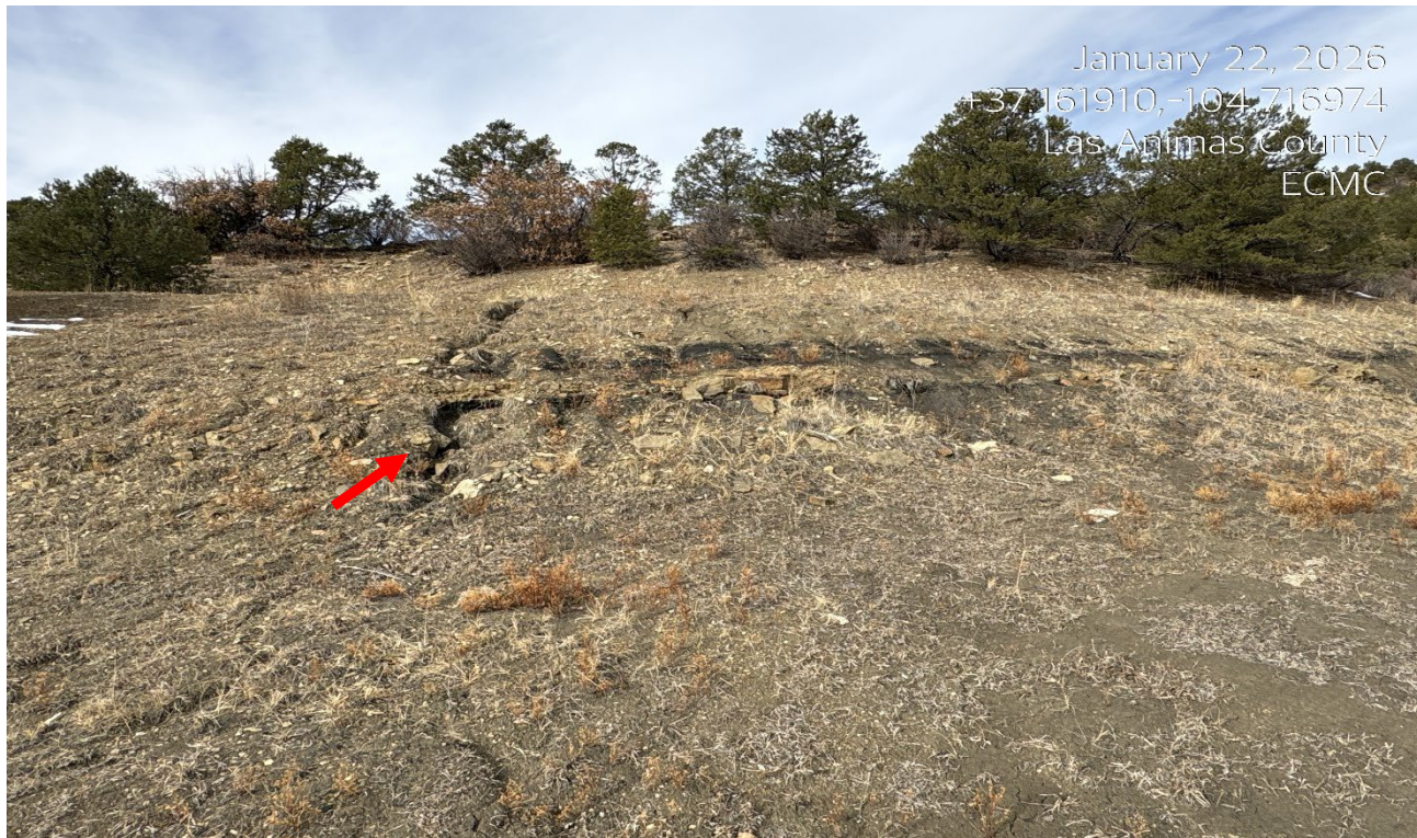
Photo 7. There is an erosion channel along the cut slope shown at red arrow.
