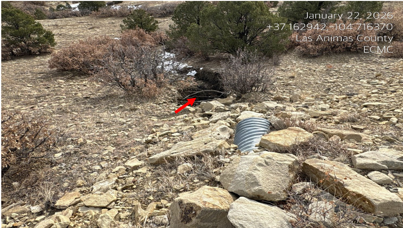
Photo 2. The culvert outlet needs additional outlet protection where erosion has occurred.
