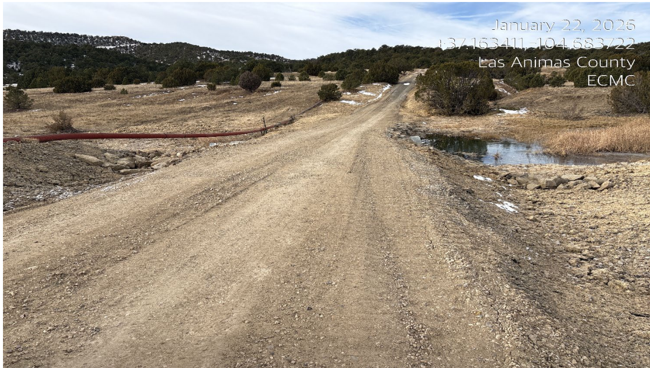
Photo 1. Facing west along the access road. There were recent repairs at the drainage crossing. Additional BMP's have been installed in this area.
