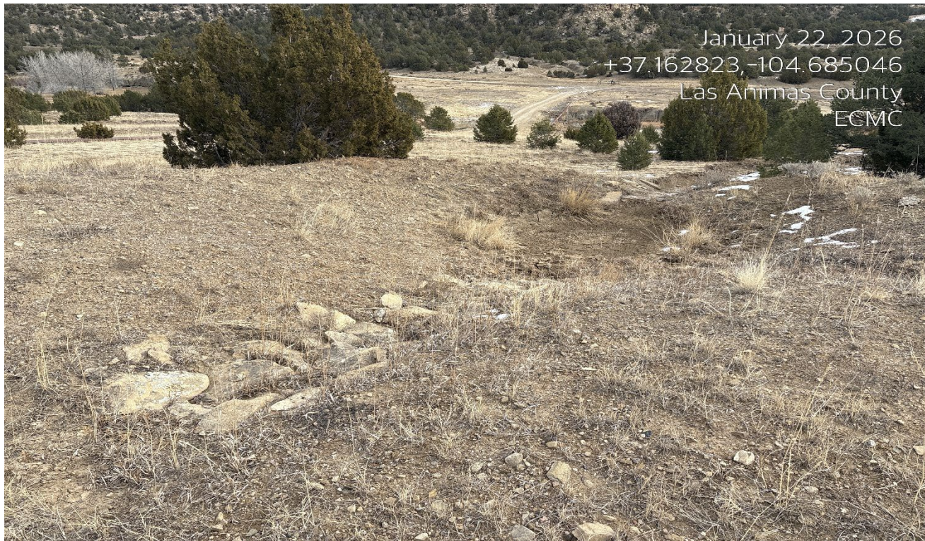
Photo 3. There is a sediment tap at the northeast corner that is maintained..
