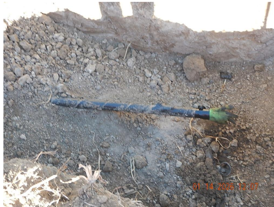
Cut end of Stonebraker 42-12 off location flowline at western endpoint. The cut end appears to be capped; work glove has been placed over the pipe cut end Stained soils can be seen under cut end of pipe
