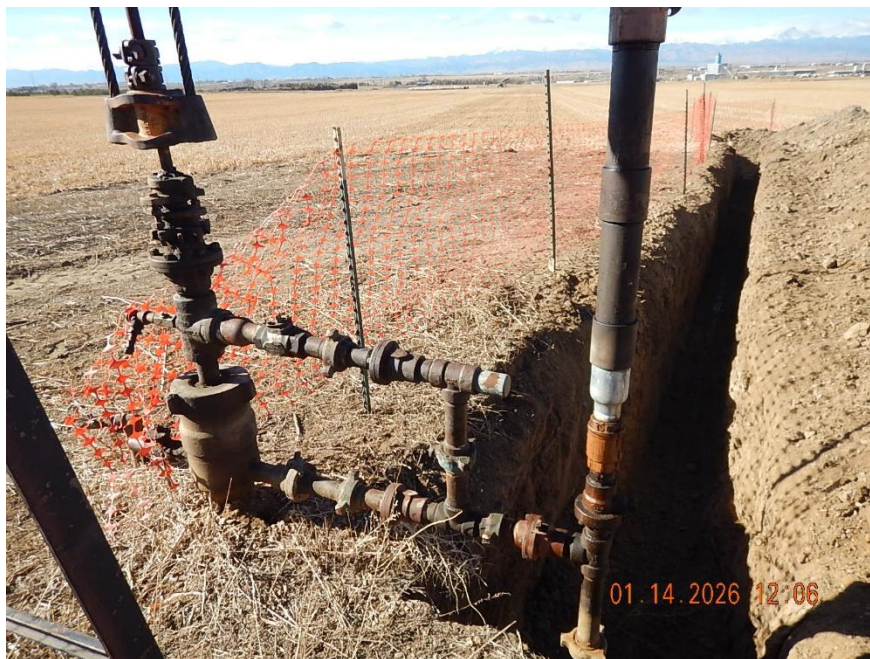
Wellhead and flowline manifold; valves are SI No OOSLAT observed in place on flowline valves at wellhead Flowline trench open from wellhead approx. 100' to west
