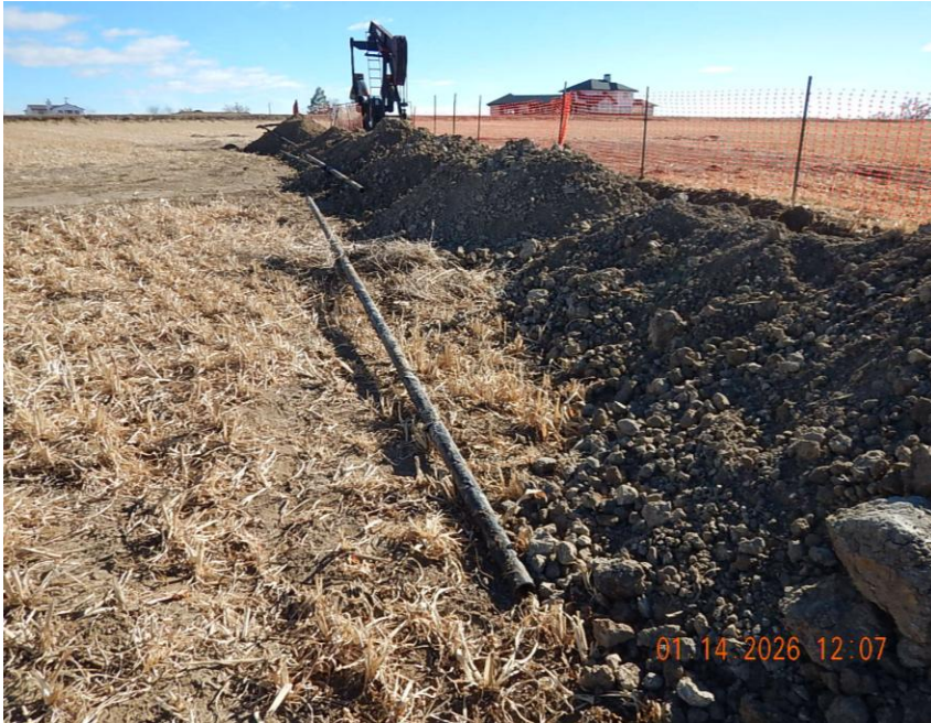
Flowline pipe segment removed; 2" carbon steel off location multiphase flowline with historical tape wrap external coating View looking east
