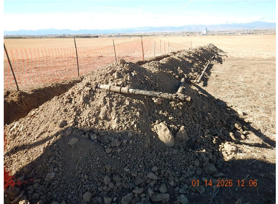
Flowline pipe segment removed; 2" carbon steel off location multiphase flowline, 90 elbow and flowline riser that previously tied into wellhead manifold. View looking west
