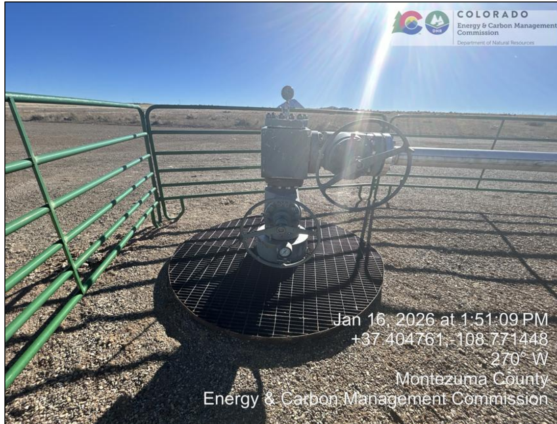
03. Well head assembly. Bradenhead is visible below grate in cellar.
