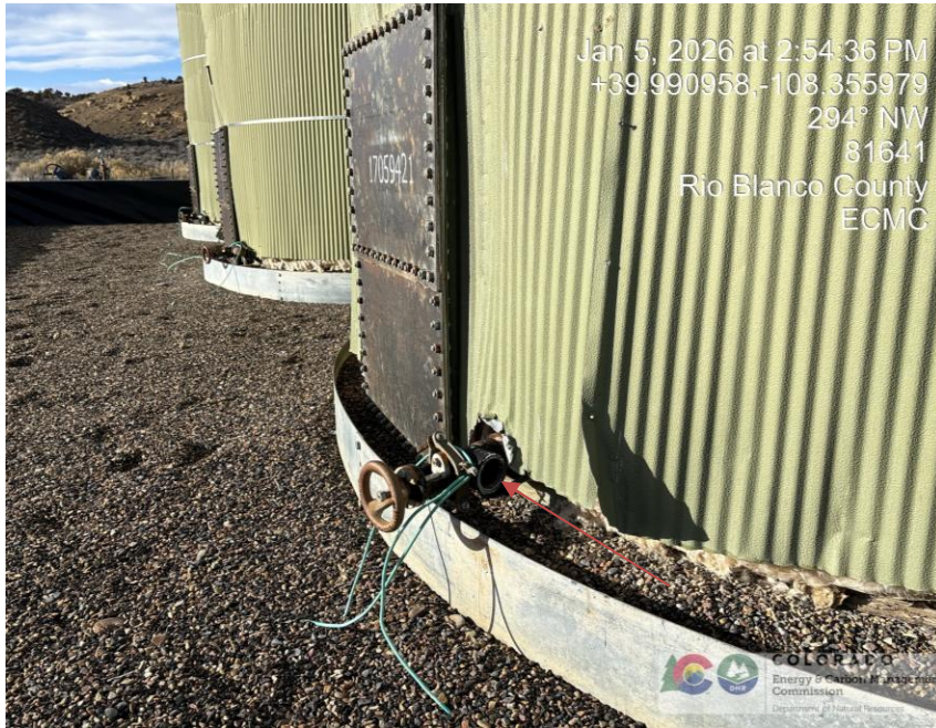
Photo # 0546 Open ended load line
