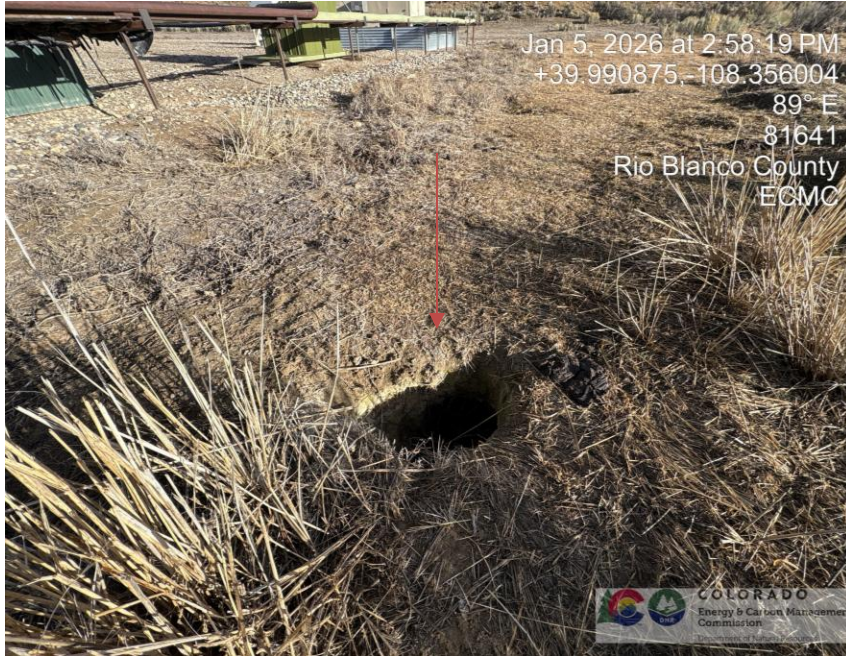
Photo # 0552 Tunnel erosion on south side of location
