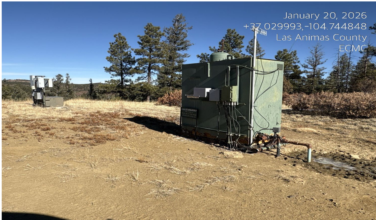
Photo 3. Facing toward the meter shed. Sign is posted at meter shed.
