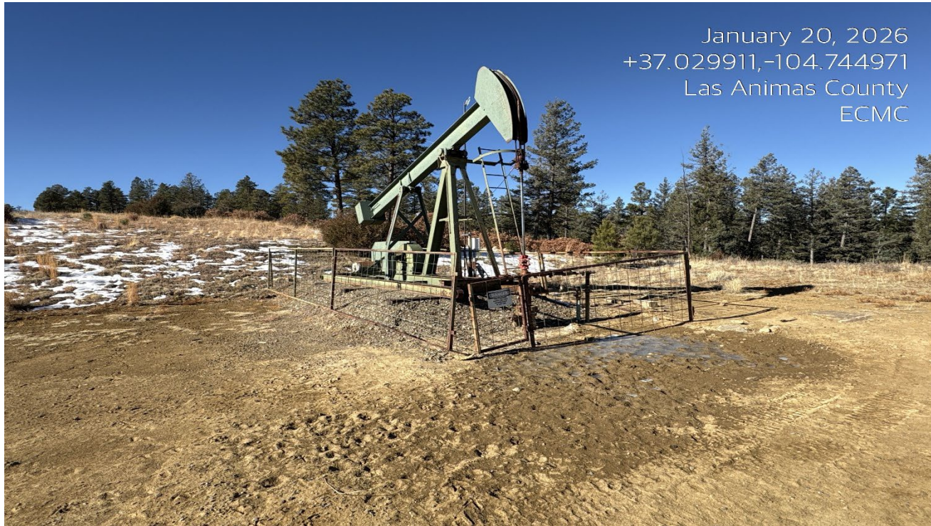
Photo 2. Facing toward the pumpjack.
