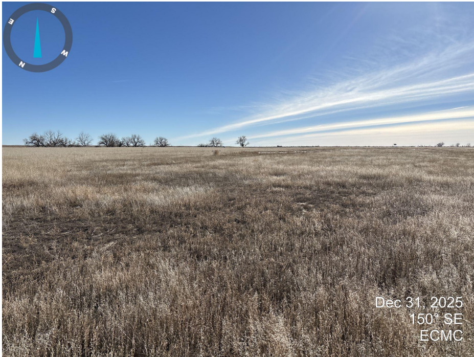
Photo 11. Looking south across the tank battery location and access road. There appears to be slight depressions/subsidence on the tank battery location.
