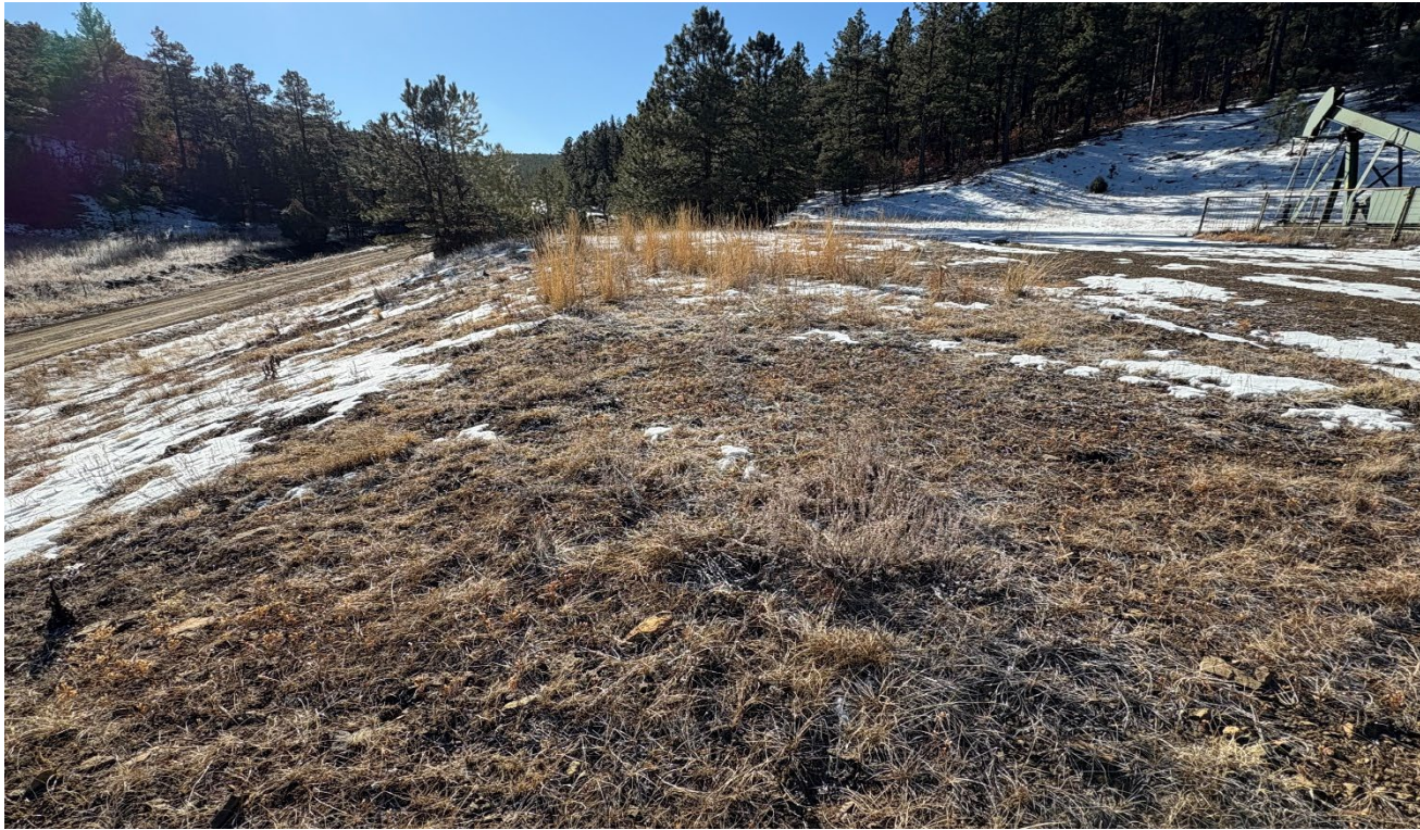
Photo 3. Facing toward the fill slope of the location which is stabilized with vegetation.
