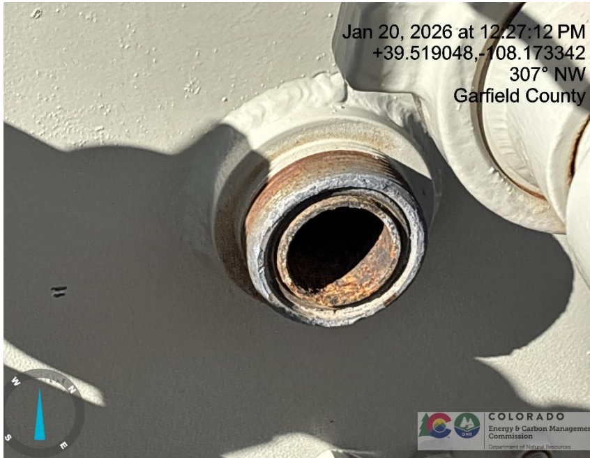
Photo # 2827 Choke body on separator open ended/wildlife hazard
