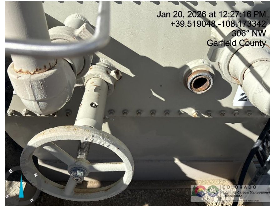
Photo # 2826 Choke body on separator open ended/wildlife hazard
