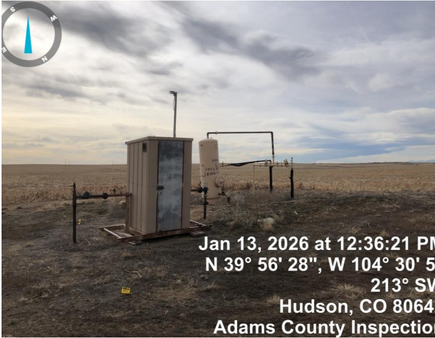
PHOTO#3 GAS METER/VERTICAL SEPERATOR
