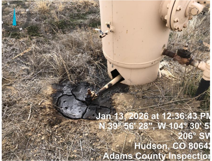
PHOTO#4 VERTICAL SEPERATOR LEAKING
