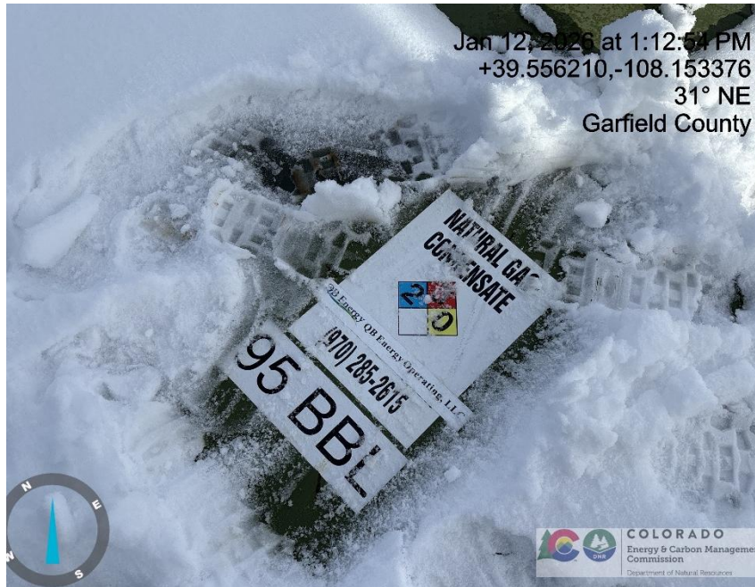
Photo # 97 Labeling on partially buried tank
