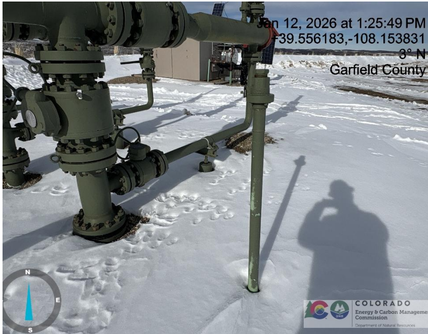
Photo # 101 Unused flowline lacks lockout tagout (OOSLAT)
