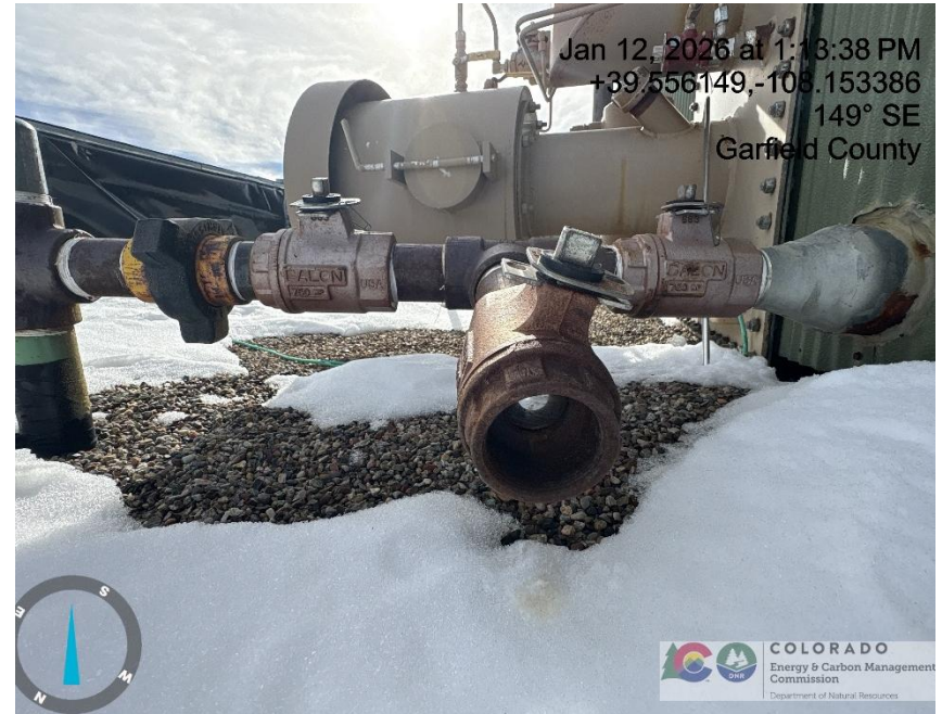
Photo # 94 Open ended load line
