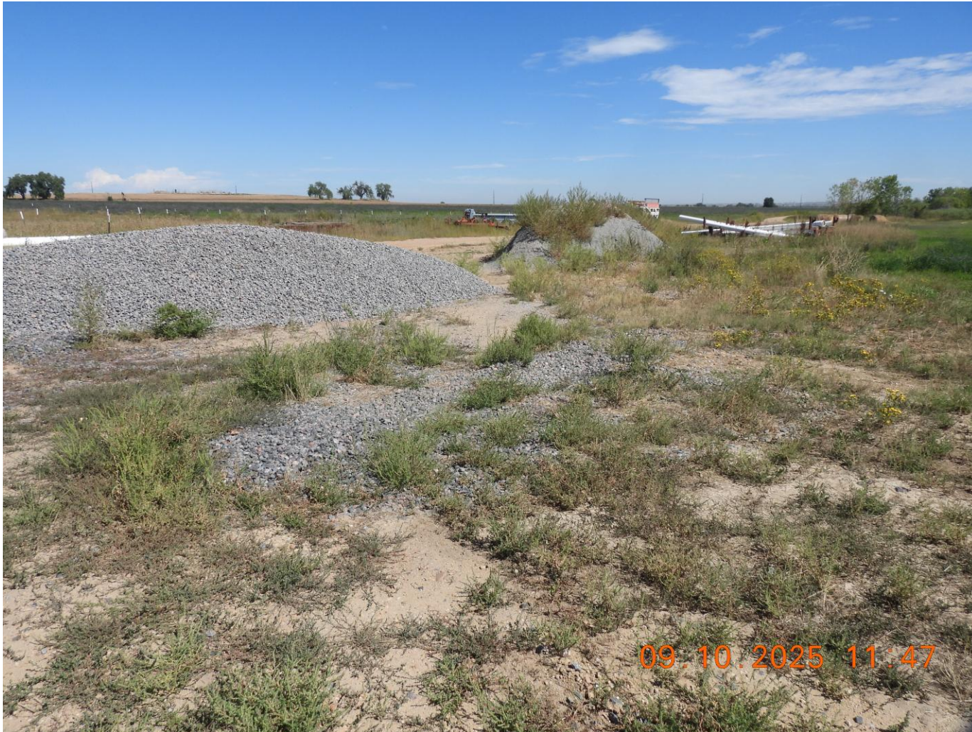
Photo 17. Ground imagery taken from the tank battery location (displaying the gravel pile).
