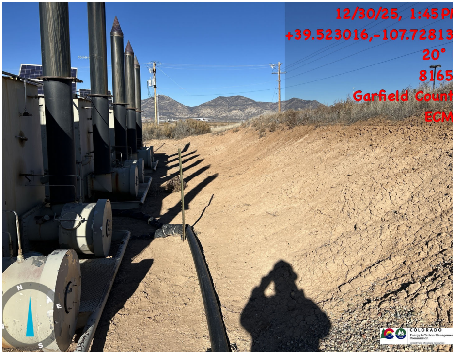
Cut slope erosion
