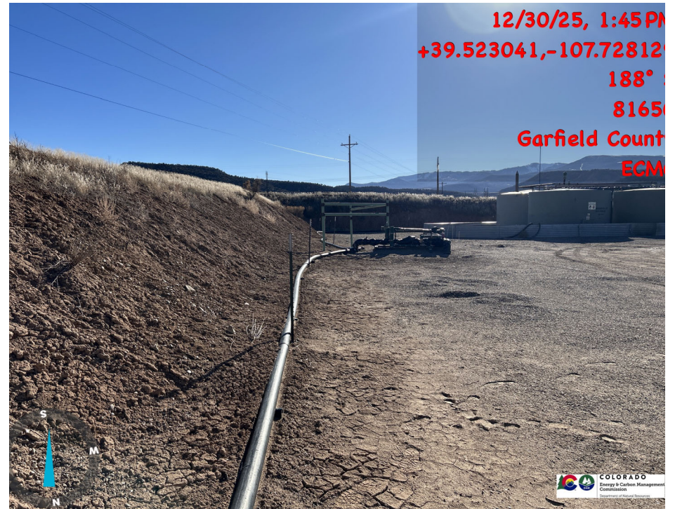
Cut slope erosion
