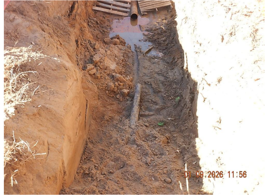
KPK Facility #2 consolidation off location flowline exposed in excavation. (1) 8 " CS and (1) 4" HDPE pipe/ material were observed in the excavation. The flowline transition area has been cut out in preparation for repair (view looking west)
