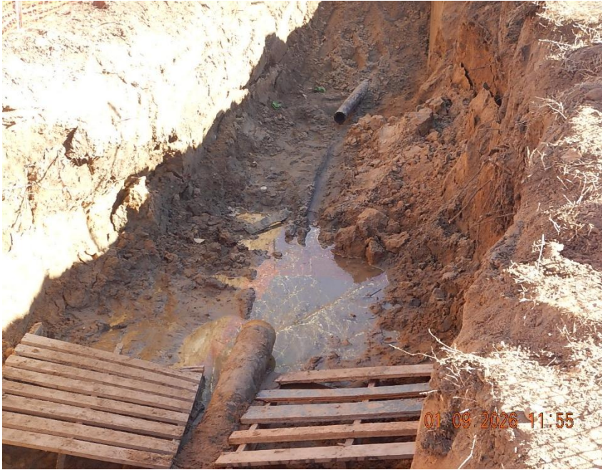
KPK Facility #2 consolidation off location flowline exposed in excavation. (1) 8 " CS and (1) 4" HDPE pipe/ material were observed in the excavation. The flowline transition area has been cut out in preparation for repair (view looking east)
