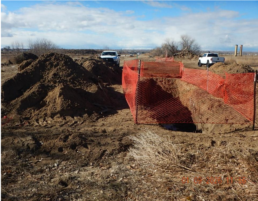
Fenced excavation exposing facility #2 consolidation line at area of failure. Inspection date 1/9/26 (view looking west)
