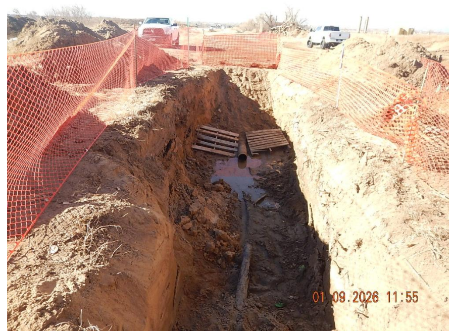
KPK Facility #2 consolidation off location flowline exposed in excavation. (1) 8 " CS and (1) 4" HDPE pipe/ material were observed in the excavation. The flowline transitions from 8" CS (to west) to 4" HDPE (to east) in the excavation.
