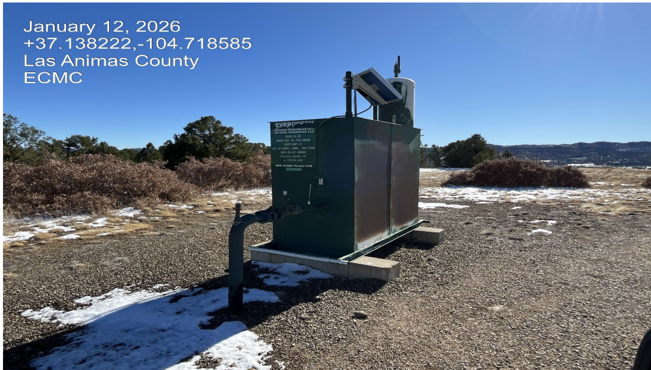
Photo 2. well sign is posted at the meter shed.
