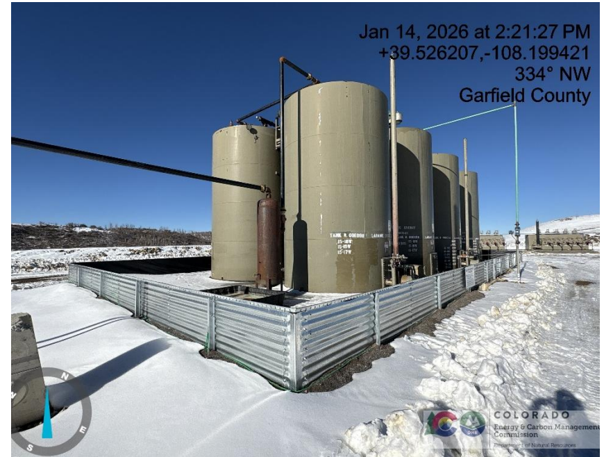
Photo # 1282 Tank battery lacks required signage
