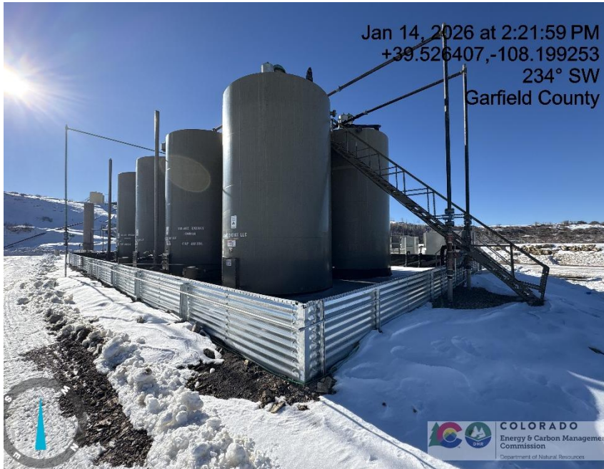
Photo # 1283 Tank battery lacks required signage
