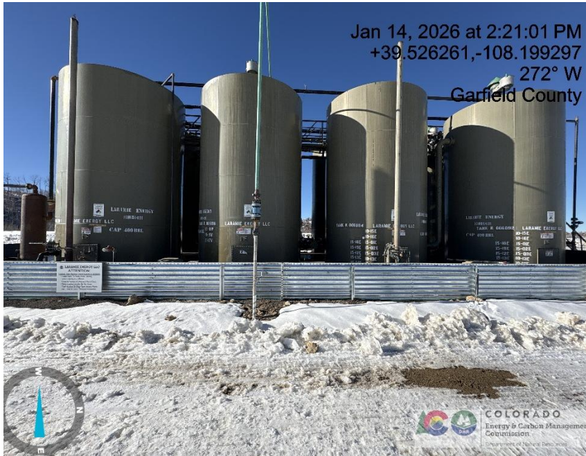
Photo # 1281 Tank battery lacks required signage
