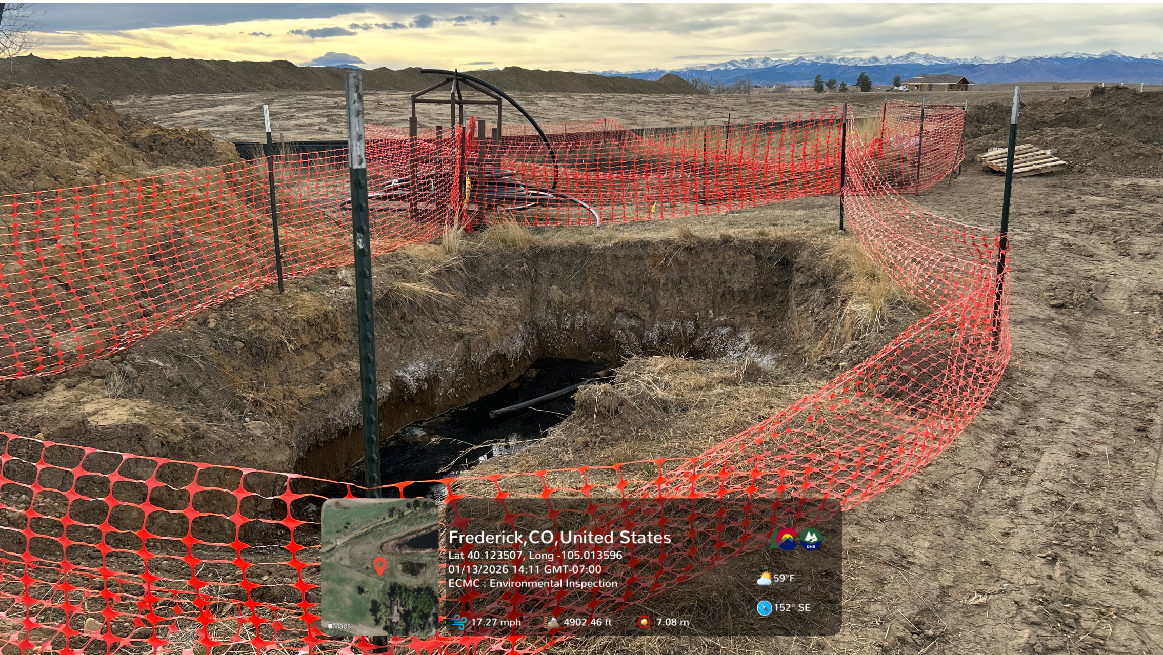
Looking at both excavations at the spill location. Orange construction fencing surrounds the eastern excavation but is beginning to fall.
