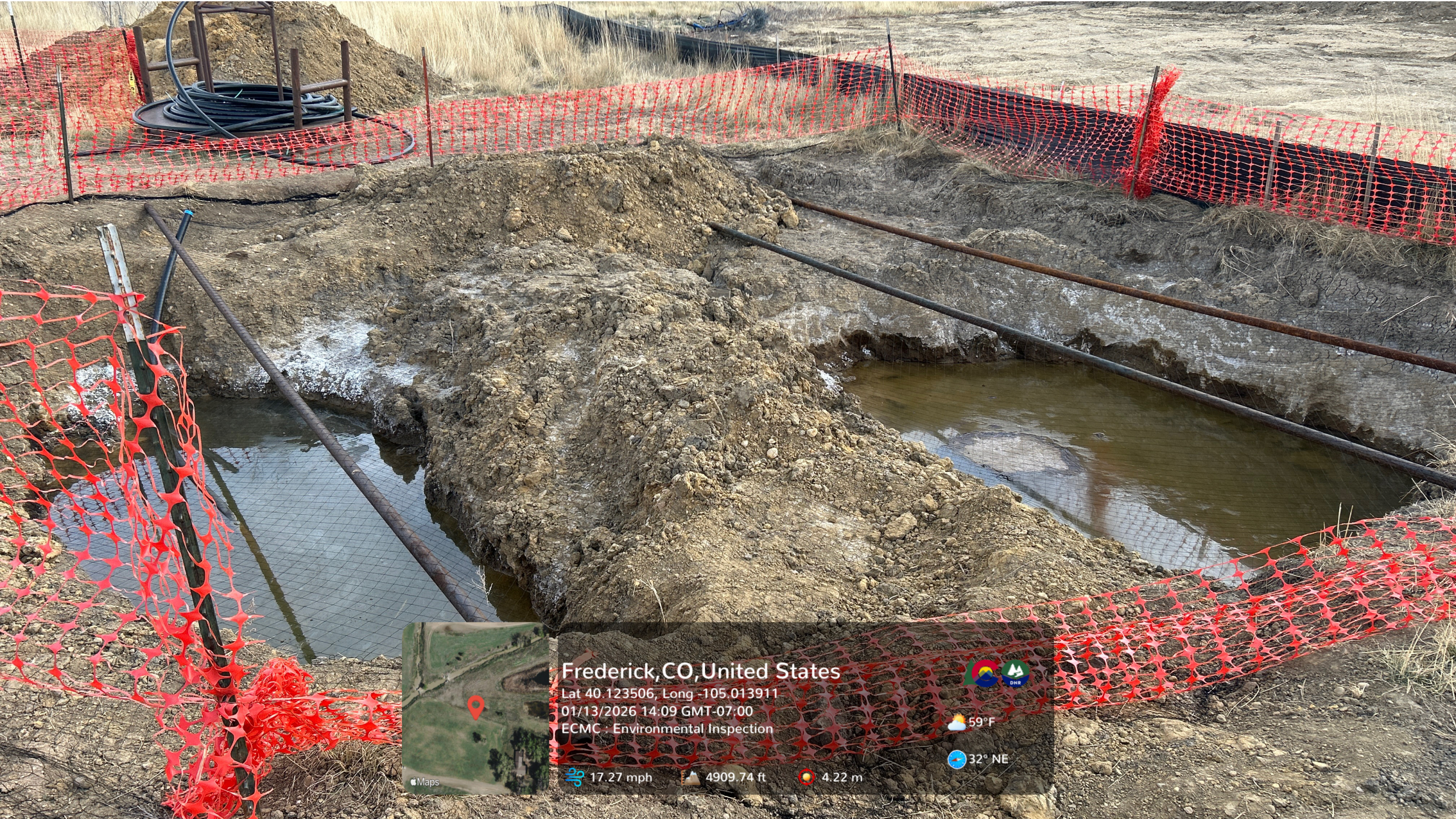
Looking at the northern and southern excavations open at the spill location. Petroleum hydrocarbon saturated soil, stained soil, and salt crusting are visible on the excavation sidewalls. A sheen and free product are visible on groundwater at the base of the excavations. Bird netting has been installed over the open excavations.
