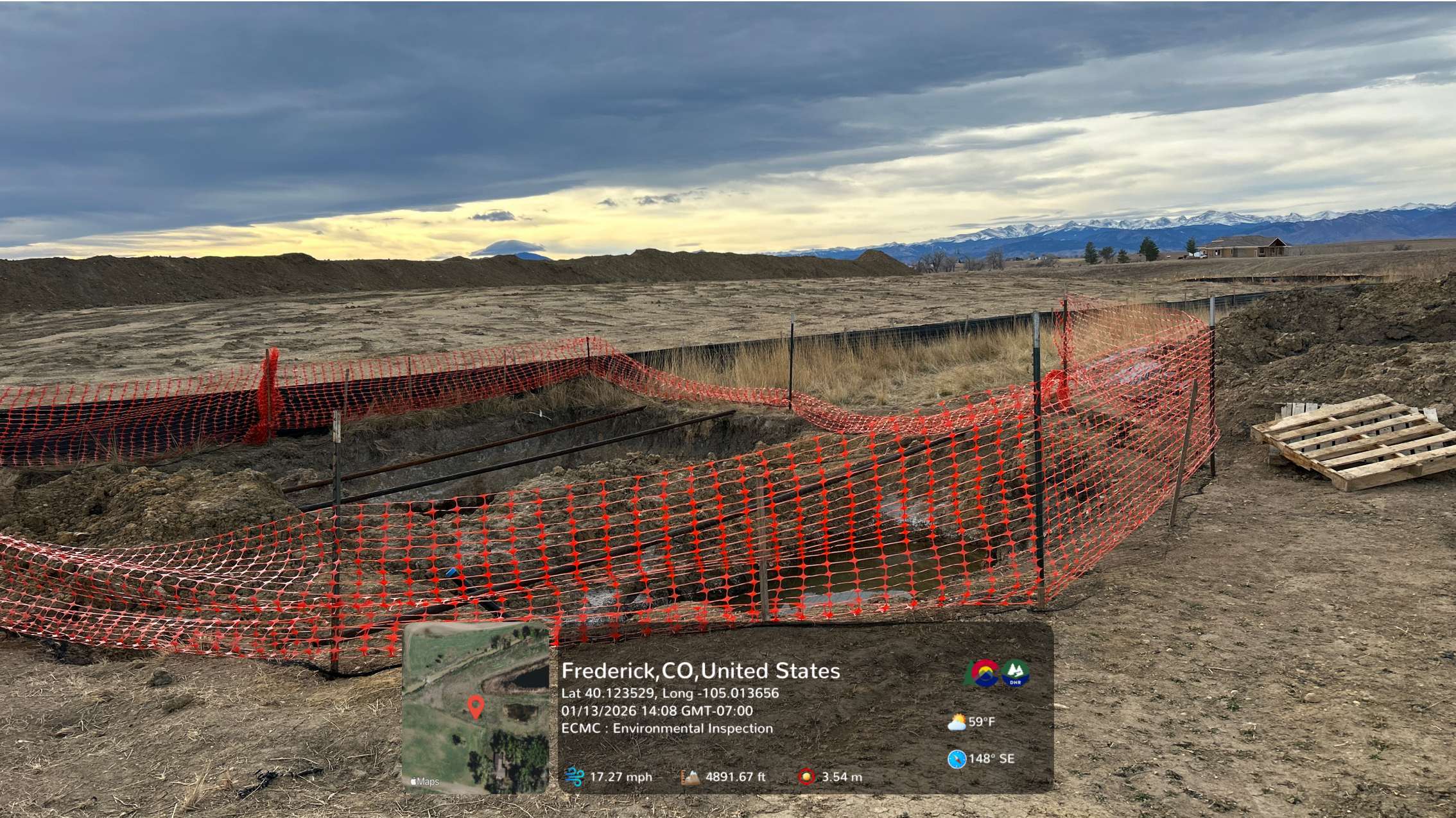
Looking at the spill location. Orange construction fencing has been installed around the open excavations, but has fallen.
