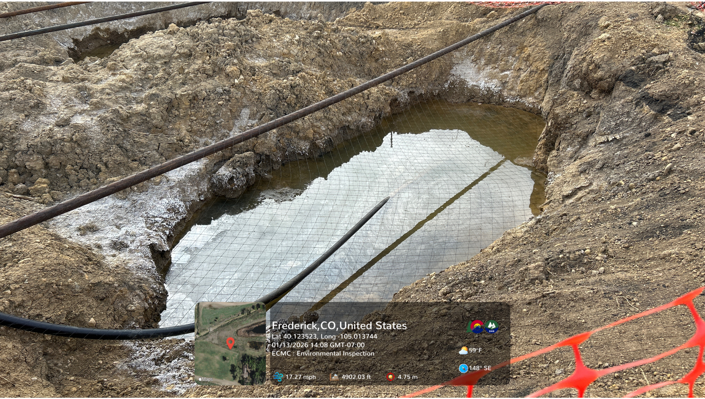
Looking at the northern excavation open at the spill location. Stained soil and salt crusting are visible on the excavation sidewalls. A sheen is visible on groundwater at the base of the excavation. Bird netting has been installed over the open excavations. A segment of flowline is visible protruding from the excavation.
