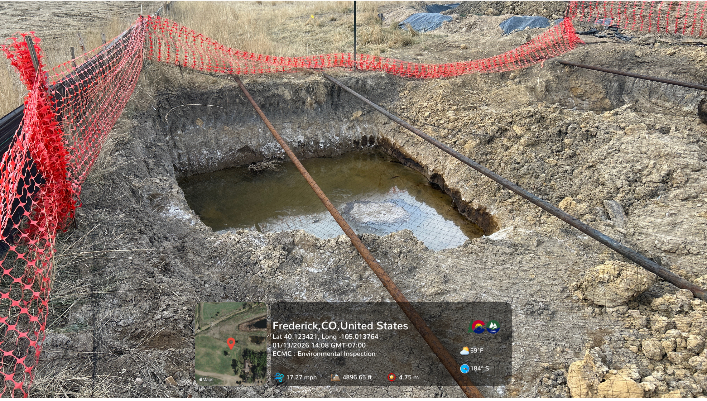
Looking at the southern excavation open at the spill location. Petroleum hydrocarbon saturated soil and salt crusting are visible on the excavation sidewalls. Free product is visible on groundwater at the base of the excavation. Bird netting has been installed over the open excavations.
