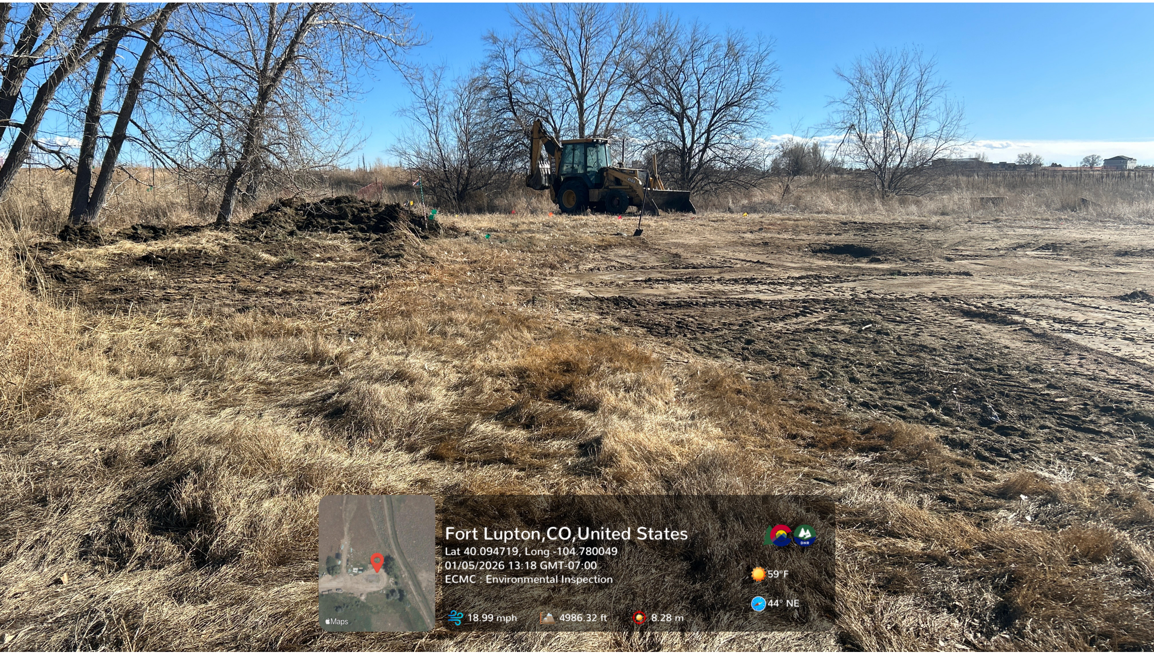
Looking east at the point at which fluid was observed daylighting from the subsurface.
