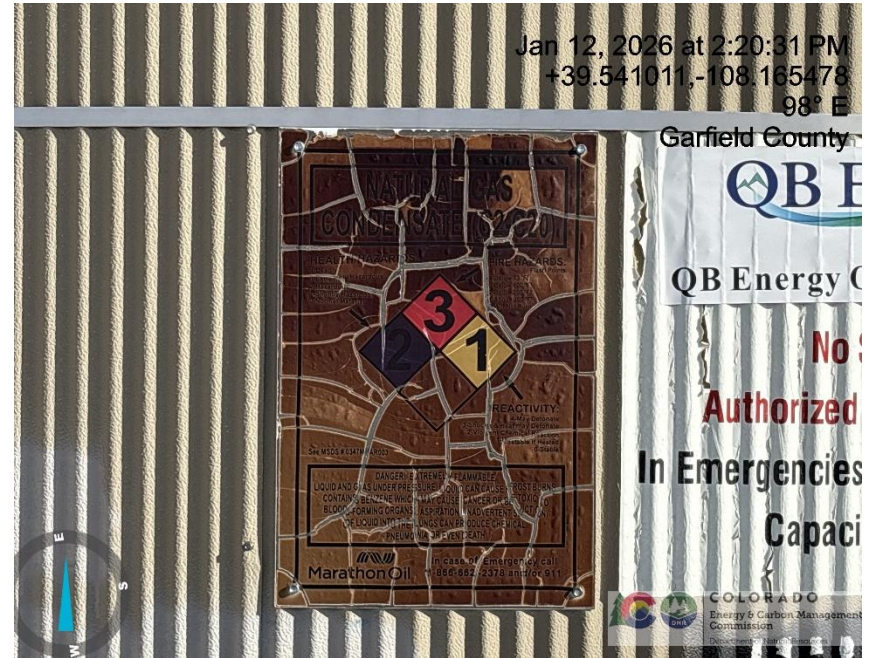
Photo # 308 Tank label damaged & illegible
