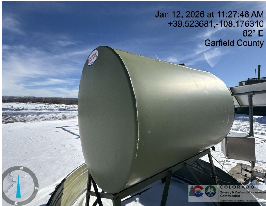
Photo # 9806 Methanol tank lacks required info
