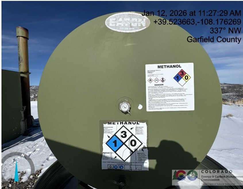
Photo # 9804 Methanol tank lacks required info
