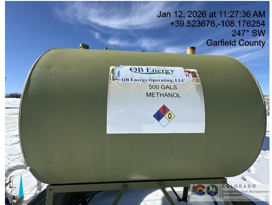
Photo # 9807 Methanol tank lacks required info
