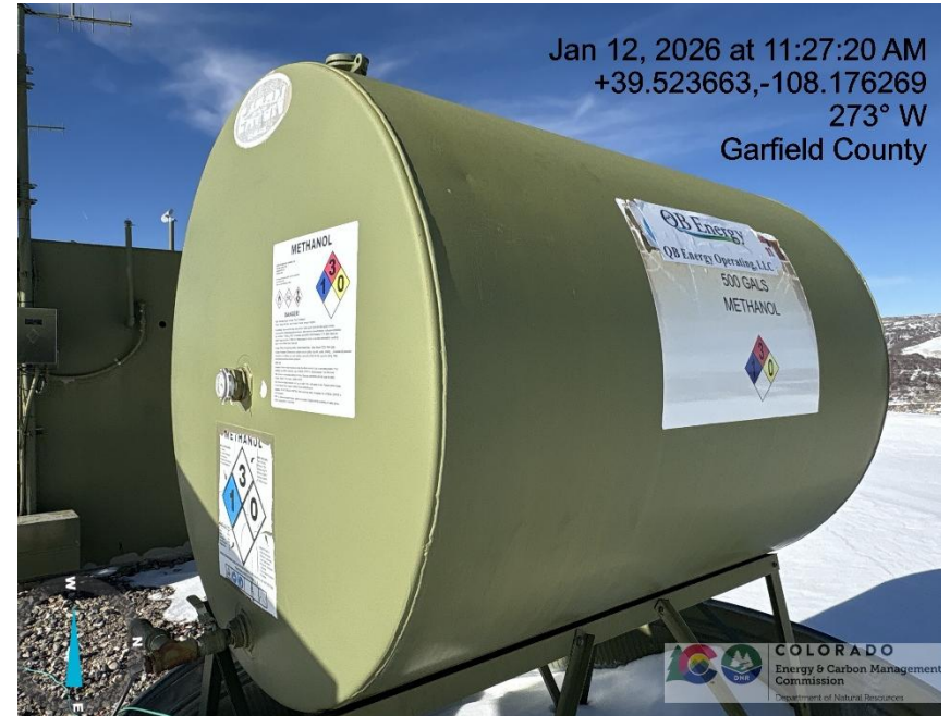
Photo # 9805 Methanol tank lacks required info
