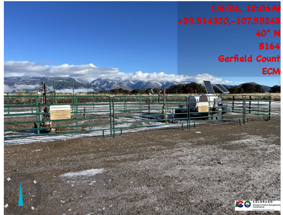
Wells and some signs are becoming illegible
