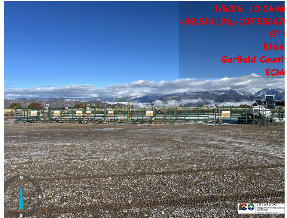
Wells and some signs are becoming illegible
