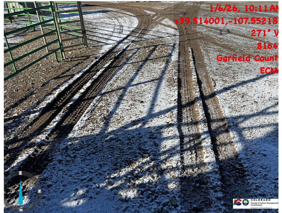
Lack of stabilization
