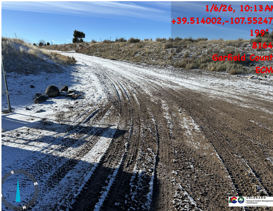
Lack of tracking/stabilization
